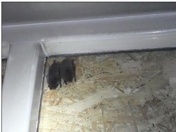
Photo 13: Two common pipistrelle bats located between timber boarding and window pane at the ground floor western elevation of the building (Roost 1)
