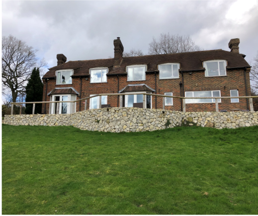
Photo 1 , Photograph looking at the existing house as seen from the rear garden. Note the retaining wall to the front that supports the amenity terrace behind.
