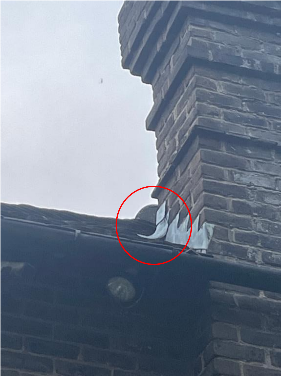
Plate 6: SE gable end chimney raised lead / wasp nest present
