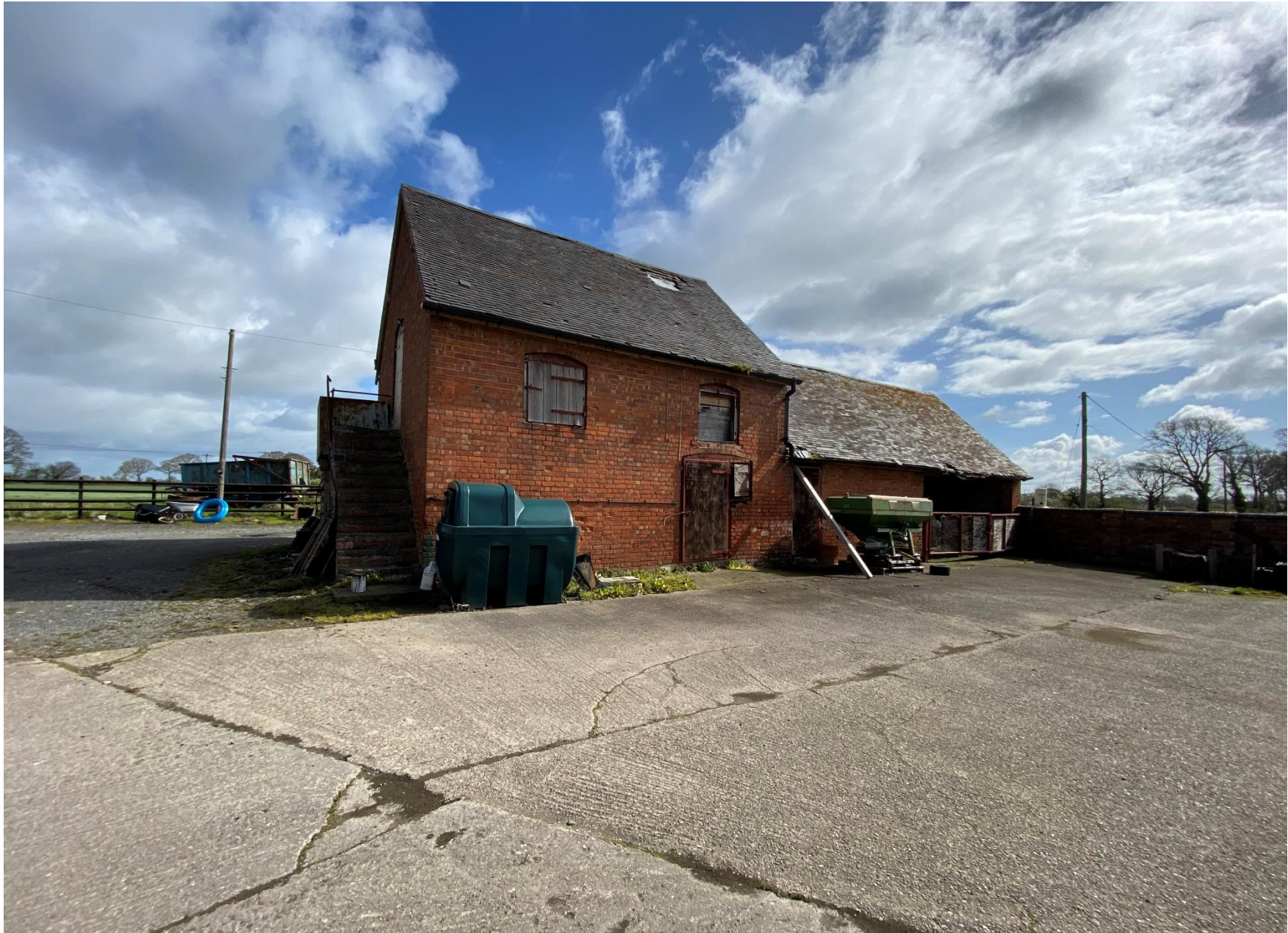
Figure 10 – Granary/Shelter Shed within Far Broadway Farmstead. Material such as oil heating container is visible.
