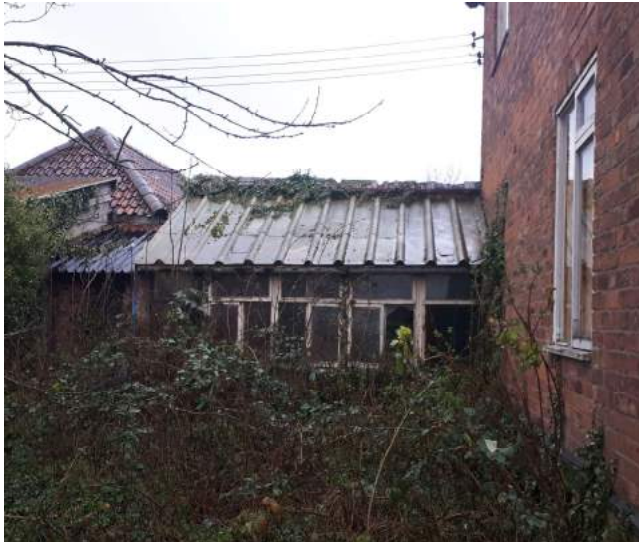
This photograph shows the wing prior to its recent demolition, with what appears to be a brickwork spine wall with capping stones
