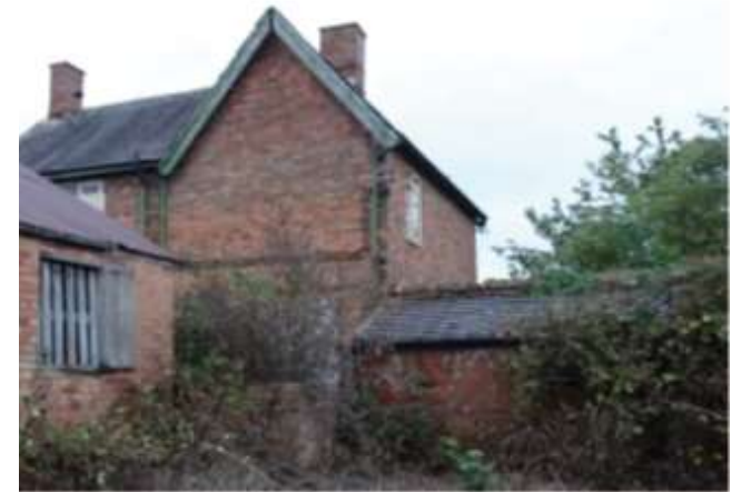
North West view of the Farmhouse with the recently demolished wing to the right of the photo
