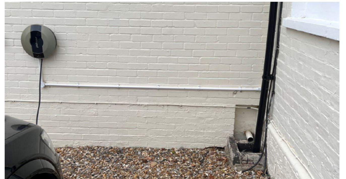
Fig 9. Picture showing the existing electric vehicle (EV) charger fixed to the East facing external wall of a rear projecting section of the Stoke Lodge building. The proposal removes the EV charger and conduit from the wall and provide a free-standing post away from the building in the corner to the right of the picture which is out of sight from the principle entrance elevation of Stoke Lodge.
