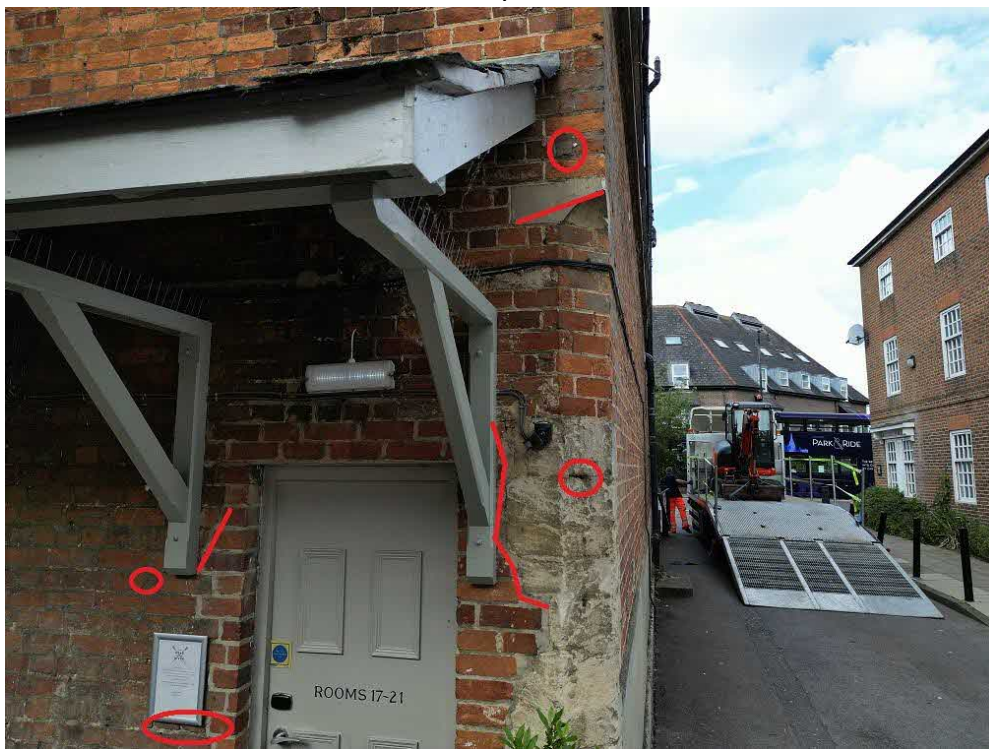
Fractures Open joints
