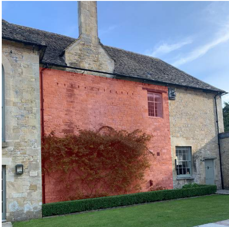
Figure 5 Detail of north front, showing replica cross casement within the wall formerly covered by the 19 th -century additions.
