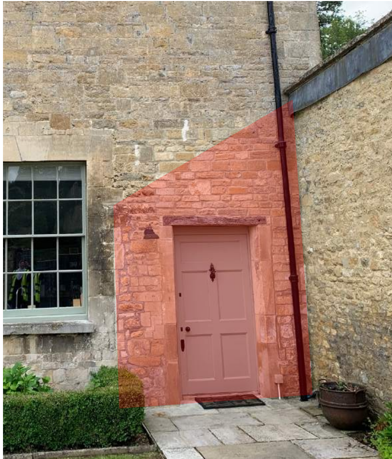
Figure 30 Detail of north elevation around the kitchen door; scar of former lean-to highlighted, lead flashing of former roof still visible beneath copings of wall to right.
