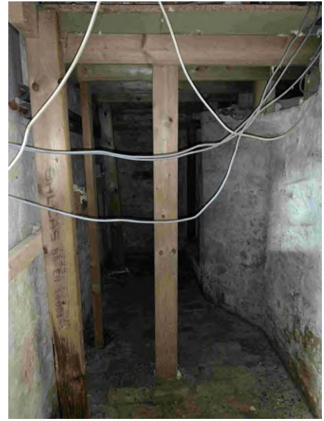
Above: View of timber supports to the chipboard floor to the Snug above.
