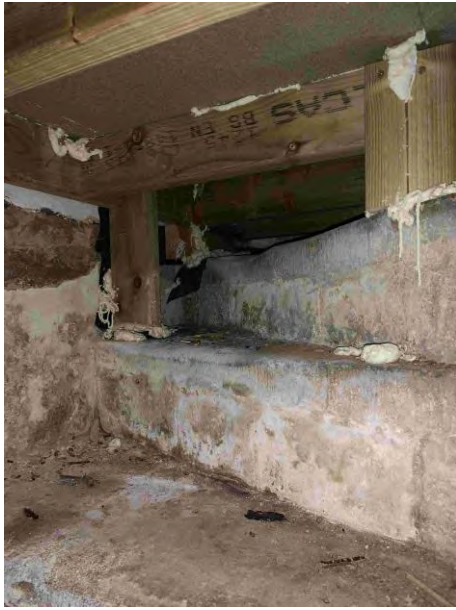
Above: View of existing spiral stair and the timber support for the chipboard floor to the Snug.
