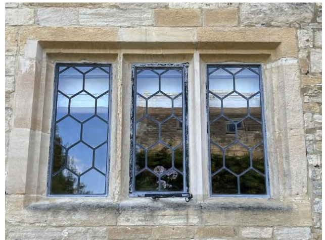
Above: Window WG26 detail. The left-hand mullion is significantly eroded, and it is proposed that this is carefully partially replaced. The right-hand mullion has already been replaced.
