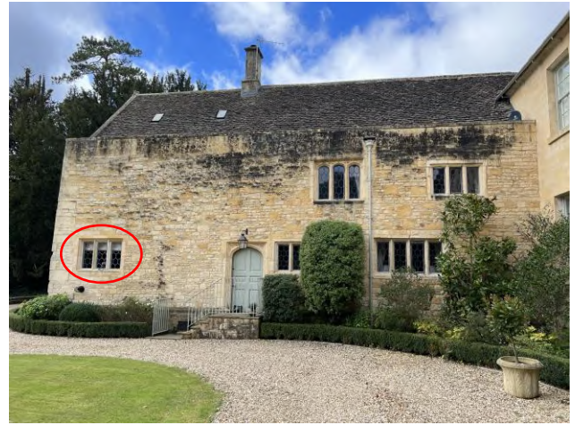
Above: West wing – east elevation as existing. The red circle indicates the affected window (WG26).
