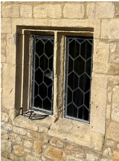
Above: Window WG31 detail. The central mullion has eroded significantly, and it is proposed that this is carefully replaced.
