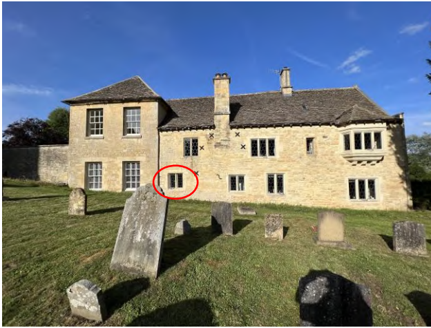
Above: West wing – west elevation as existing. The red circle indicates the affected window (WG31).
