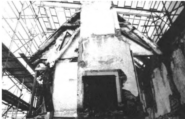
View from the Kitchen/ Parlour of the Staff Flat at the southern end of the west wing. The roof structure has been entirely removed with the parapet wall on the right hand side.
