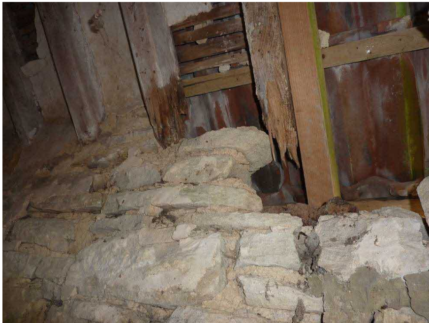
Photograph 12 Decayed rafter end bearings on to West Elevation wall.
