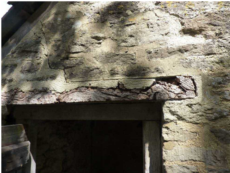
Photograph 4 Decayed timber lintel over door opening in South Elevation gable.
