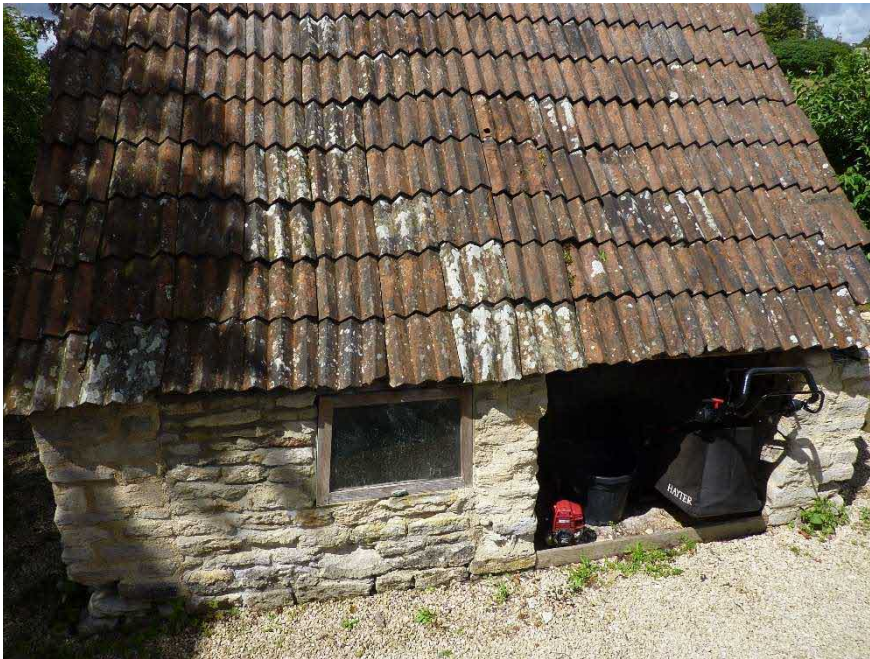
Photograph 2 East Elevation showing low eaves level and distortion in the roof structure.
