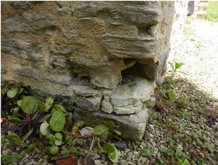
Photograph 8 Loss of low level stonework on South-East corner.
