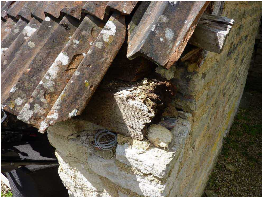
Photograph 10 Decay to timber eaves beam on North-East corner.
