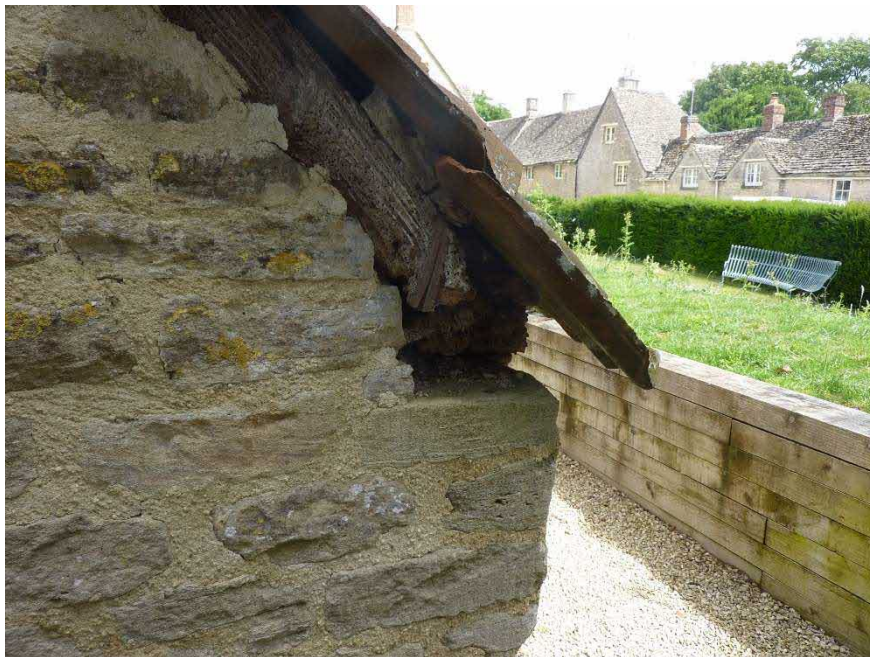
Photograph 14 Decayed verge rafter and eaves beam/wallplate on South-East corner.
