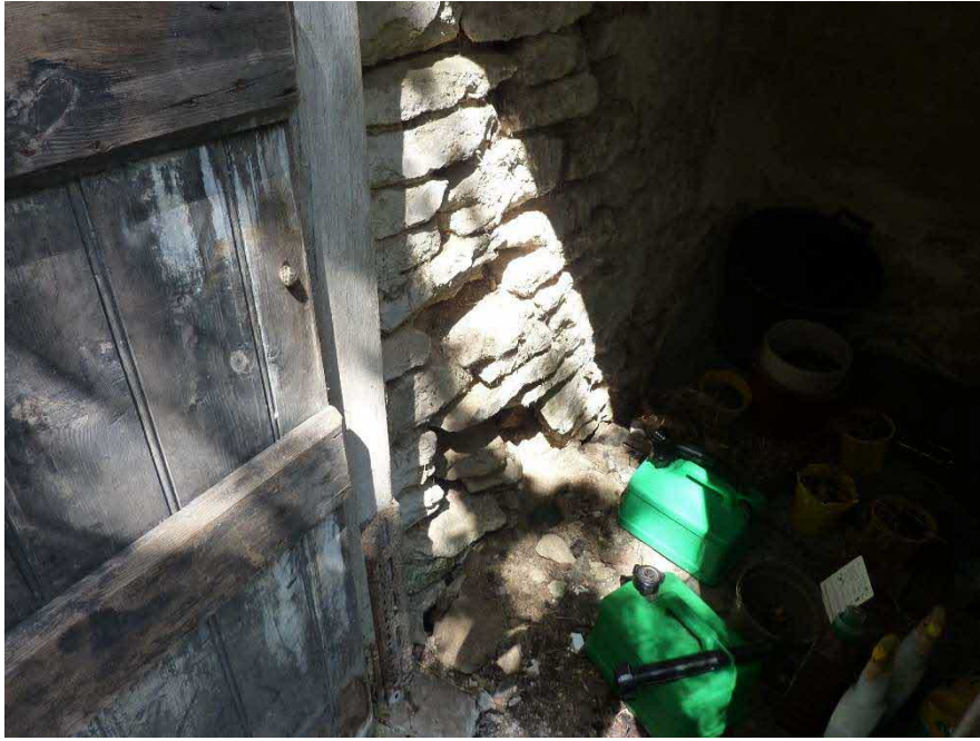
Photograph 13 Poor condition of internal wall face of West elevation adjacent to door opening.
