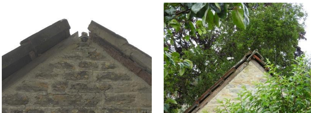
Figs. 5 & 6 Sealed south gable (L) and gaps under the roof tiles north gable (R)
