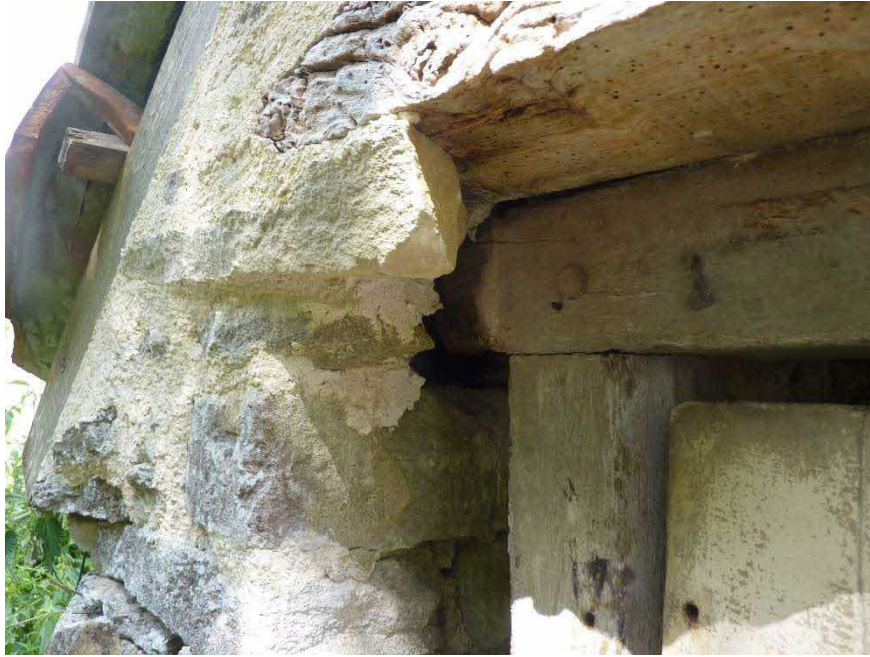
Photograph 7 Poor condition of stonework below lintel bearing on South gable.
