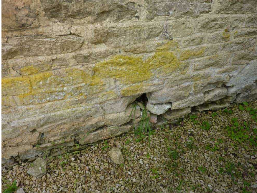
Photograph 11 Weathering of low level stonework on North Elevation gable.
