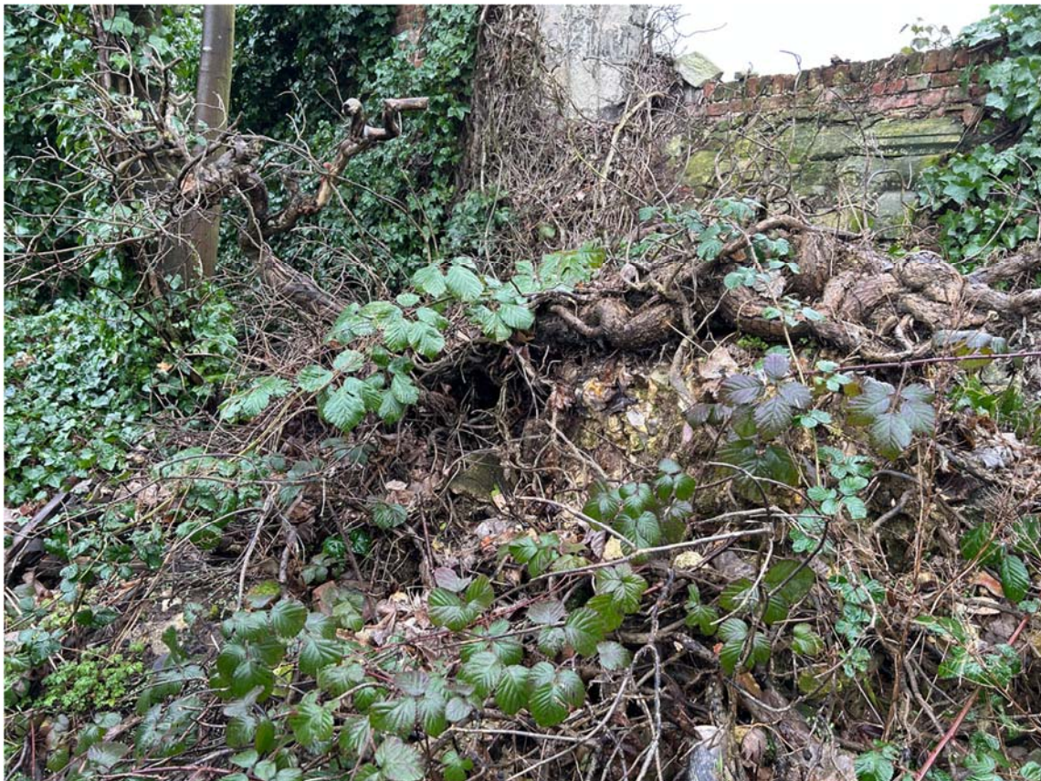
Figures 21a-c. Thoby Priory wall and remains of window arch.
