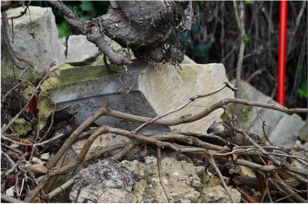
Figure 26. Fallen masonry detail
