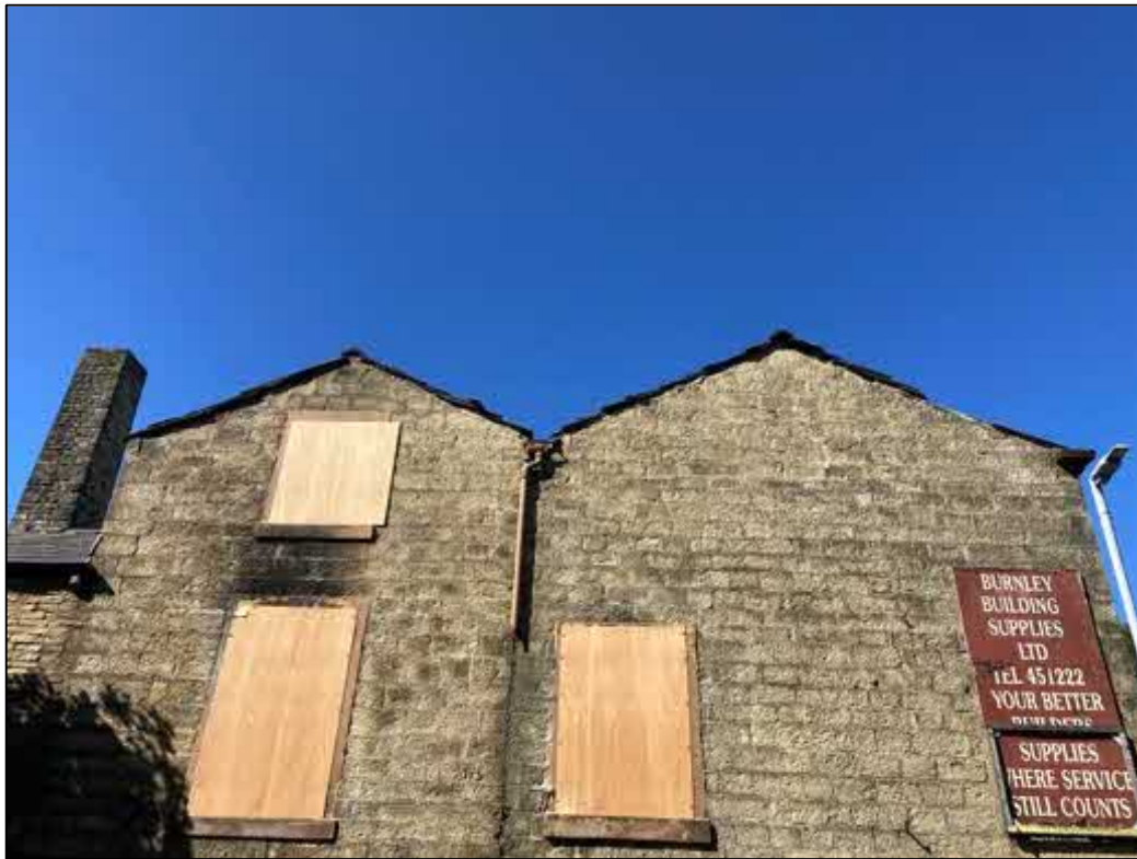
Fig 8: A view of the southern face. The twin fascia lining is in fair condition.
