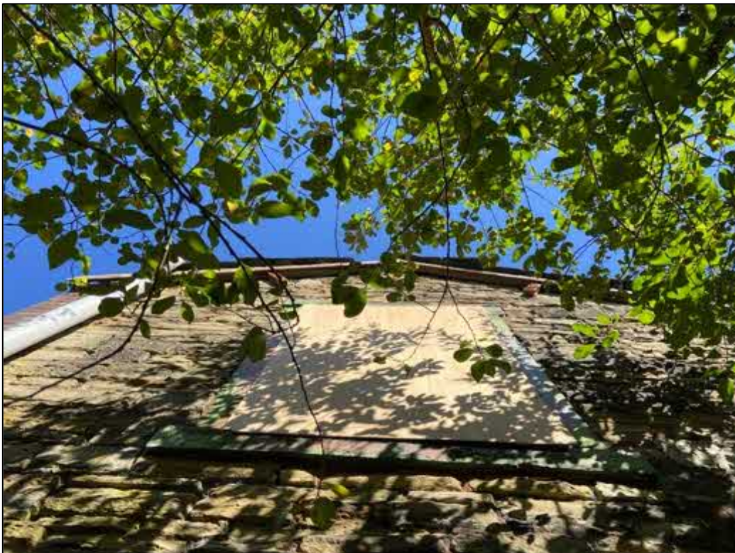
Fig 7: A view of an external wall of the building. The large brick composition creates ideal openings leading to internal wall cavities.
