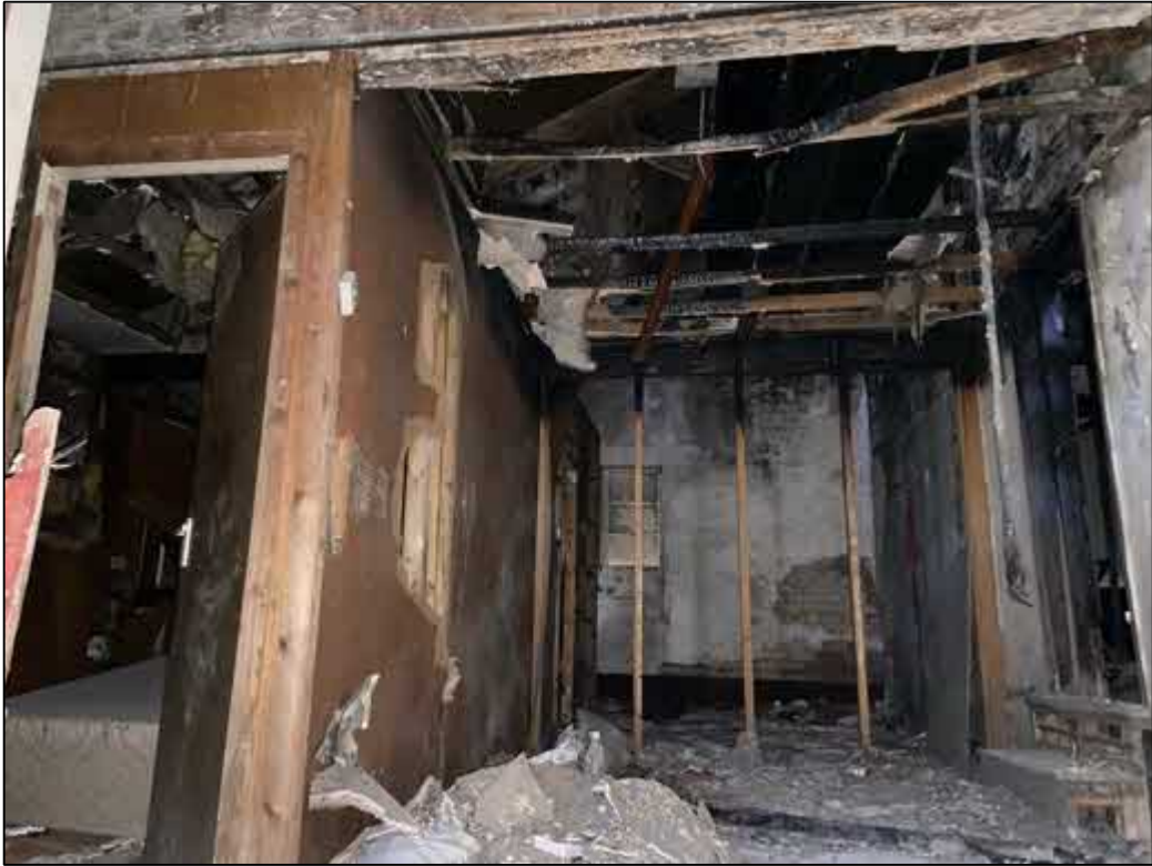
Fig 4: The upper floor of the subject building. The structural integrity of the upper floor is poor, meaning an extensive check could not be undertaken.
