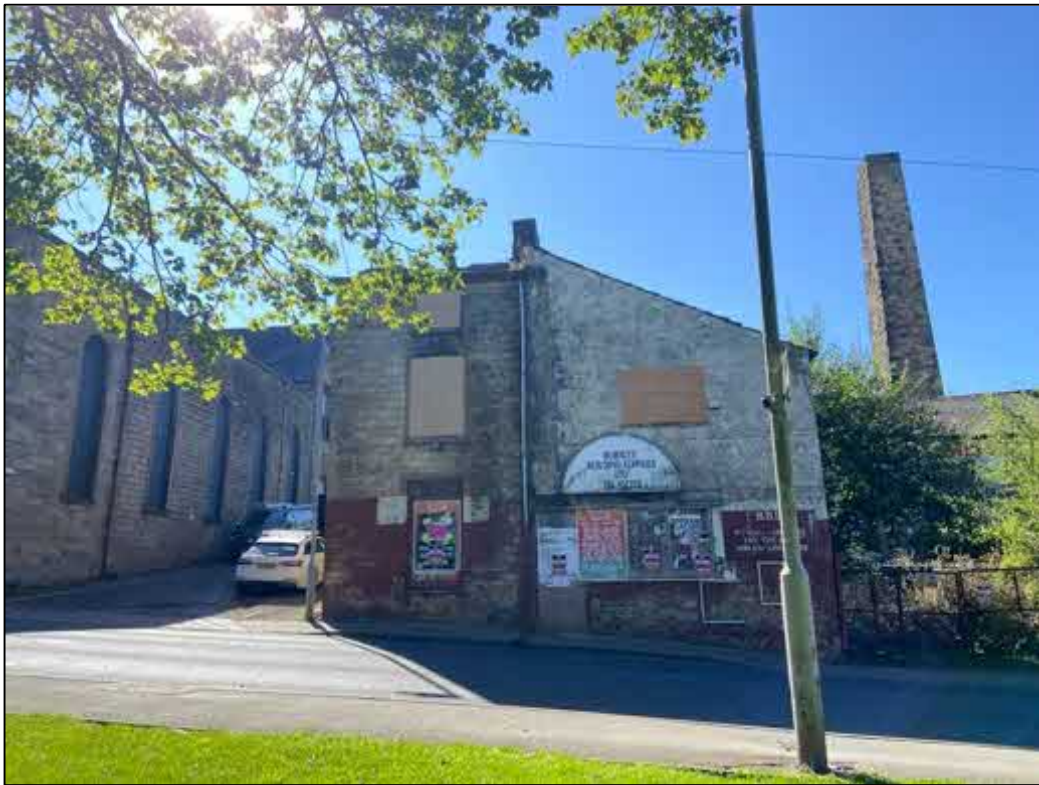
Fig 10: A front view of the subject building. The differing sections of the building can be seen. Extensive boarding across windows to deter vandalism was noted during the survey.
