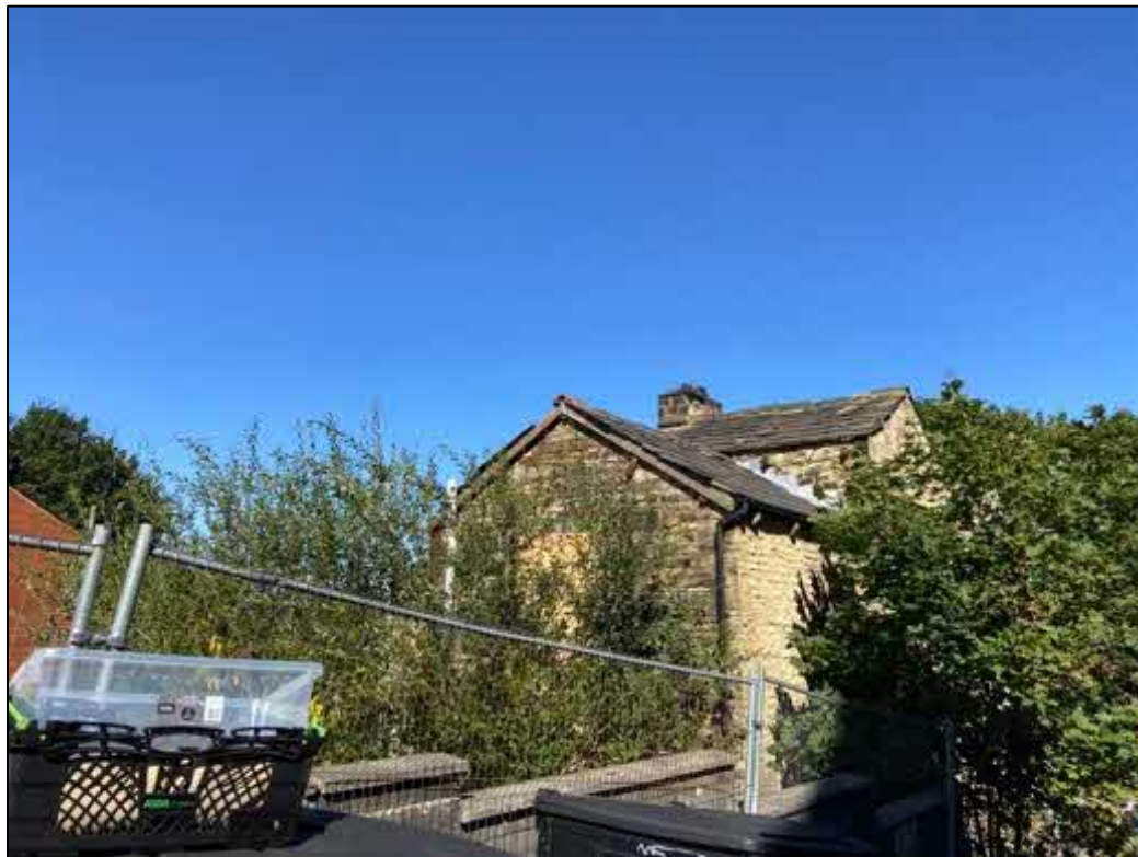
Fig 9: A further view of the rear of the building. The roof features several scattered tiles across the upper apex. The ridge lining is in fairly poor condition in places.
