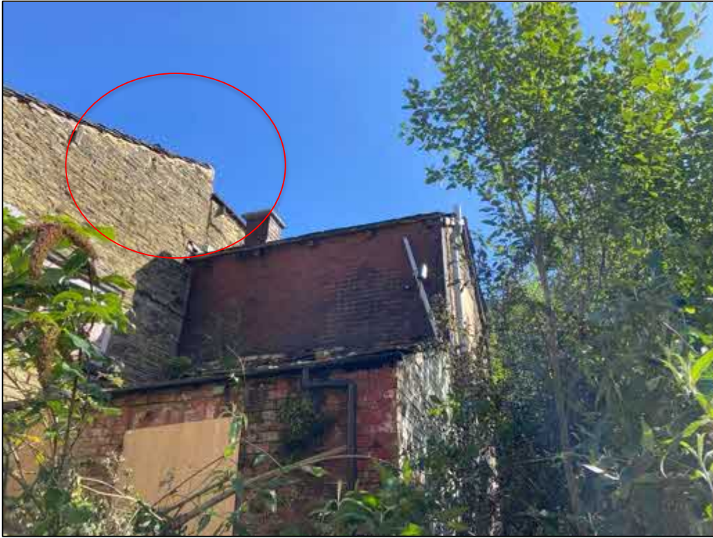
Fig 6: A closer view of the rear of the building. A differing brick section which has likely been added more recently is in fair condition. The fascia lining of the main building is in poor condition (circled).
