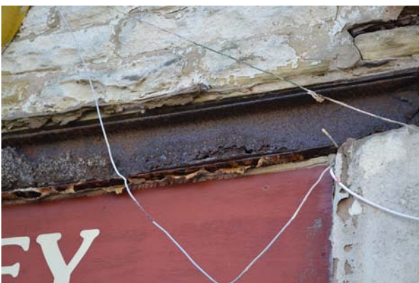
View on defect to lintel to right side wall
