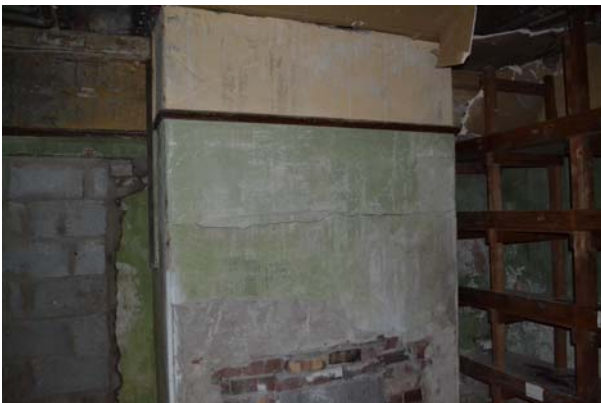
View on defects to ground floor room
