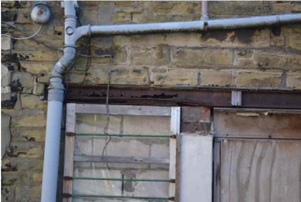
View on defect to lintel to rear wall
