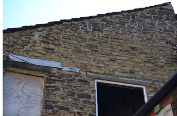
View on crack over first floor lintel
