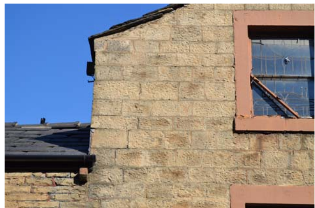
View on crack to left side elevation
