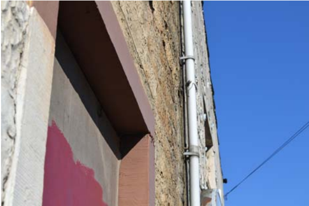
View on bulge to front elevation
