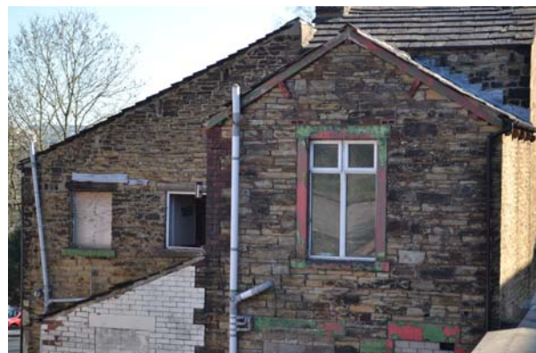
View on defects to rear wall
