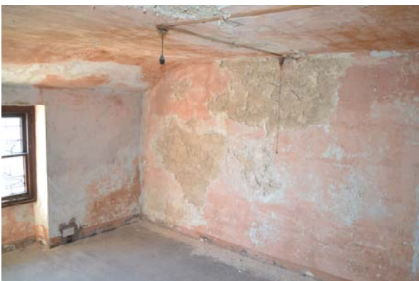
View on defects to second floor room
