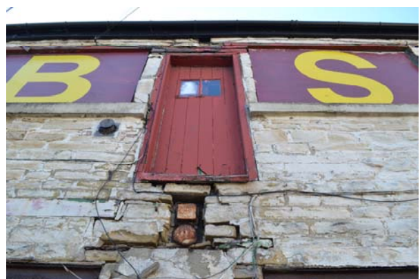
View on defects to right side wall
