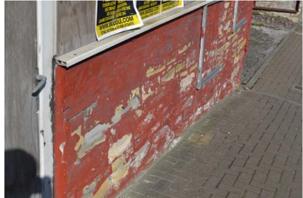
View on weathered stone to front elevation
