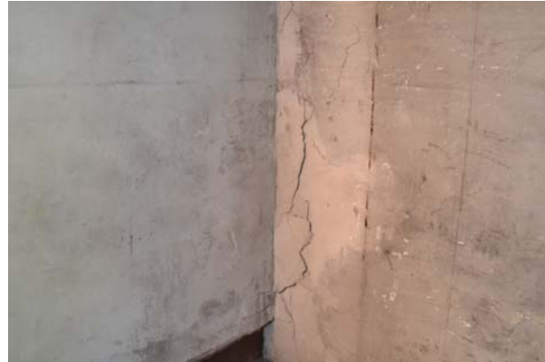
View on crack to first floor spine wall
