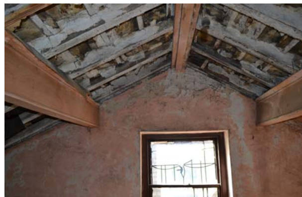
View on defects to second floor room
