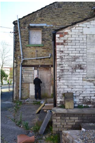
View on inclination to wall
