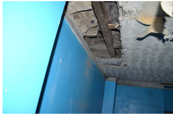
View on lack of support to chimney structure
