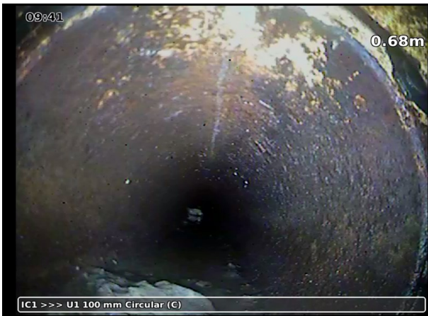
IC1X_a20c8c4d-f1f0-4193-a962-74e9b010f8c6_20230403_095800_412.jpg, 00:00:21, 0.68 m Water level, 5% of the height
