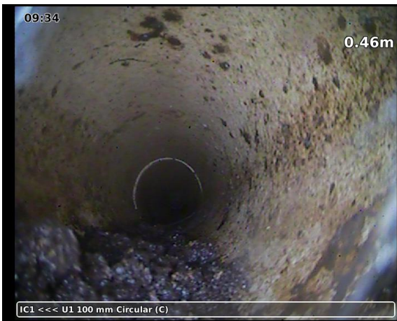
20230328-093329-snap0002.jpg, 00:00:29, 0.46 m Fine settled deposits, 5% area loss
