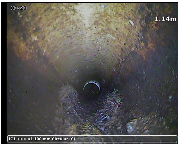
20230328-092631-snap0002.jpg, 00:02:58, 0.24 m Fine settled deposits, 20% area loss
