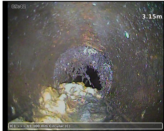
20230328-094135-snap0004.jpg, 00:01:02, 3.15 m Fine settled deposits, 20% area loss
