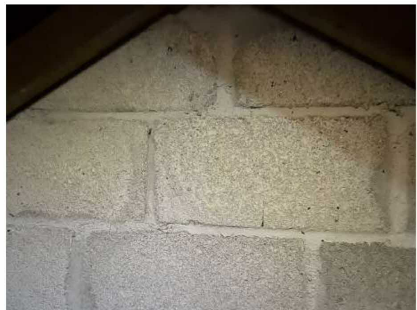
Photograph 4. Bat droppings on west gable.
