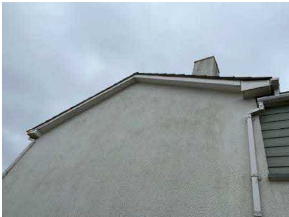
Photograph 7. Tightly fitted plastic soffits.
