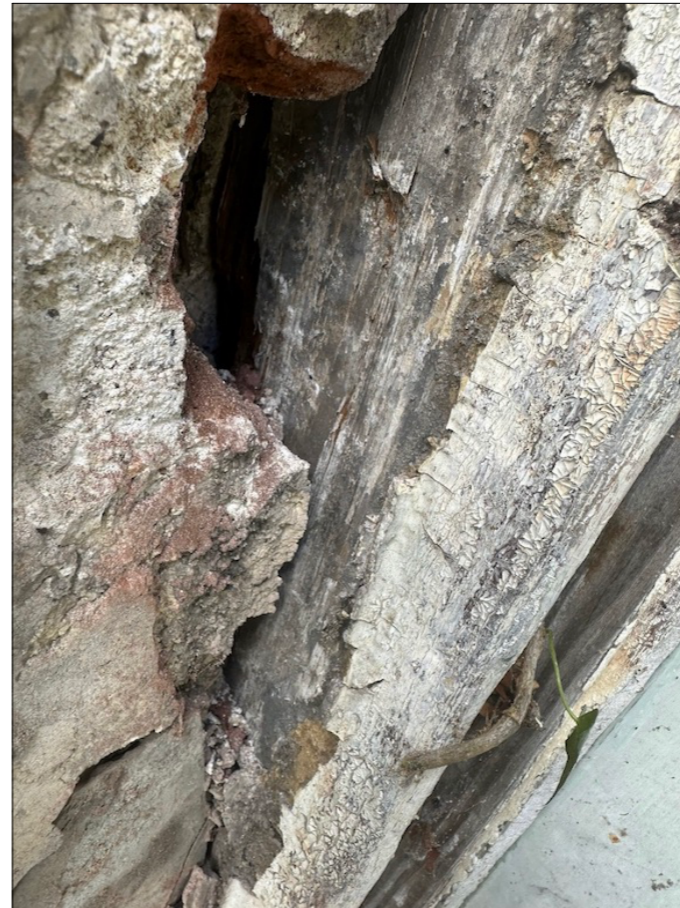
Box frames are rotten and weights have seized
