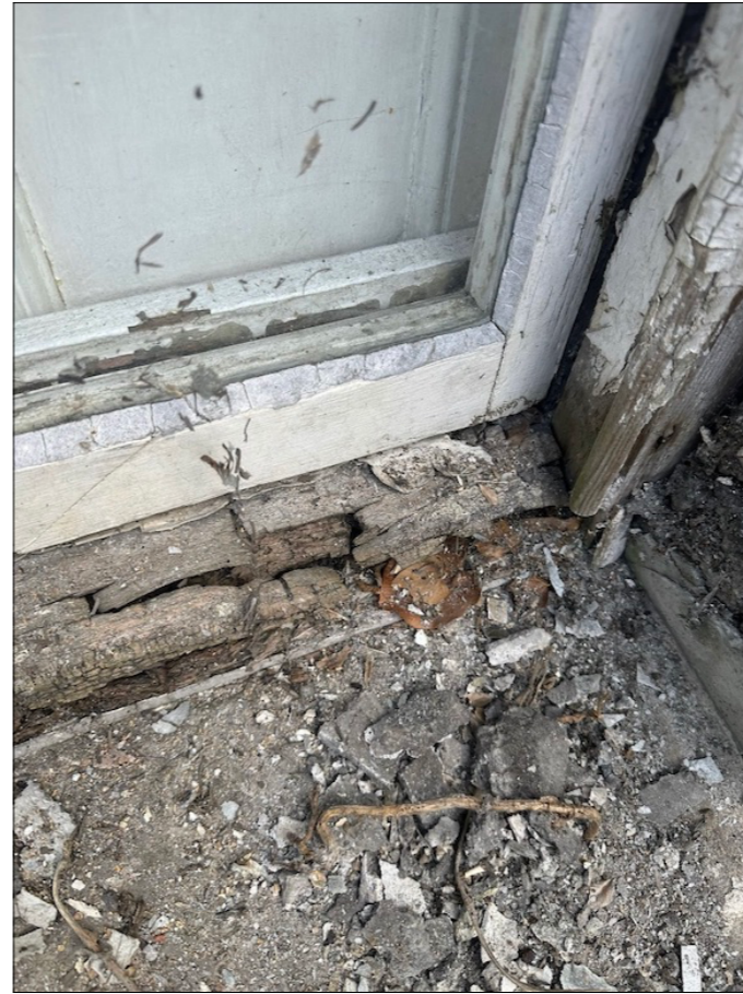
Sashes, sills, and box frames have no structural integrity
