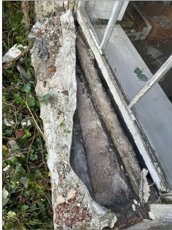
Sashes, sills, and putty are beyond repair
