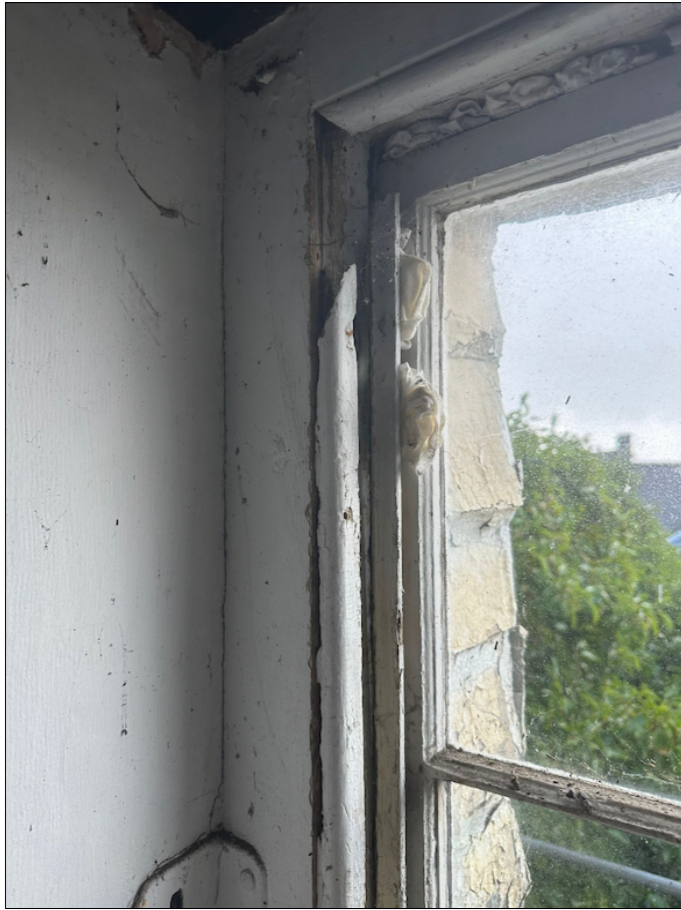
Nonfunctional sashes have been packed with tissue to reduce drafts
