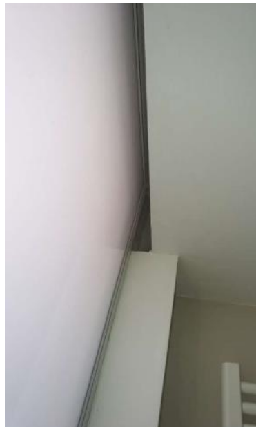
Figure 5.37: Showing the gap between the suspended ceiling and the window.
