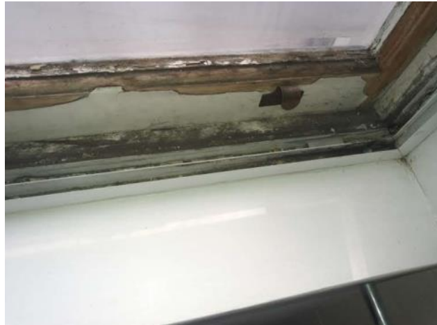
Figure 5.39: Showing the window in disrepair in the Eastern Bathroom.
