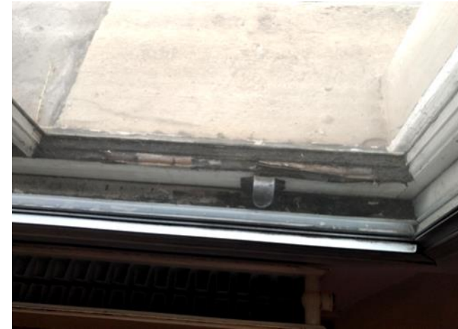
Figure 5.24: Showing the disrepair of bottom rail of the lower sash.
