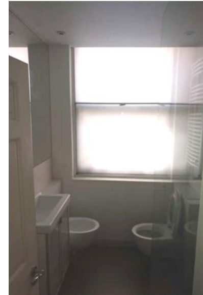
Figure 5.36: Showing the Eastern Bathroom. Note the suspended ceiling and that the top of the window is not visible.
