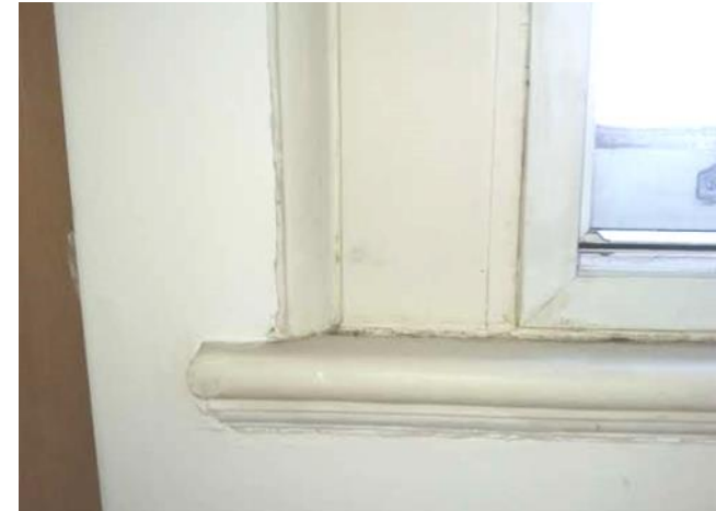
Figure 5.28: Showing the window architrave of the western wall in the Master Bedroom.
