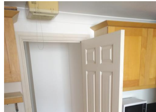
Figure 5.22: Showing the coving in the kitchen area.
