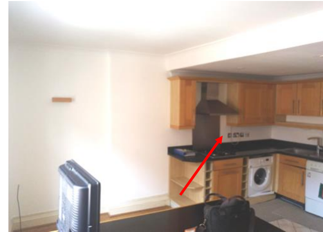
Figure 5.20: Showing the chimneybreast on the northern wall of the kitchen. The area of boxing out is shown in red.
