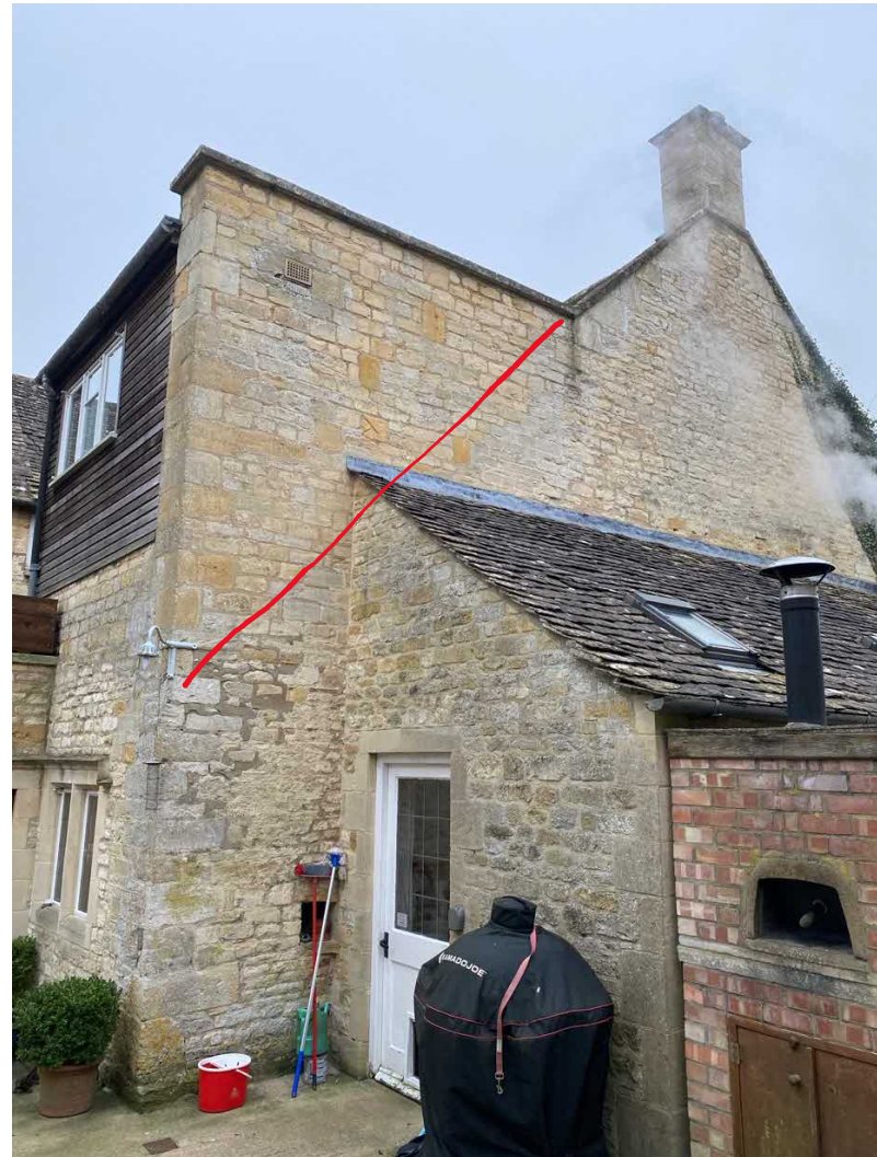
Image above showing modern 1950 bathroom extension. The masonry above the red line is part of the 1950 works.
