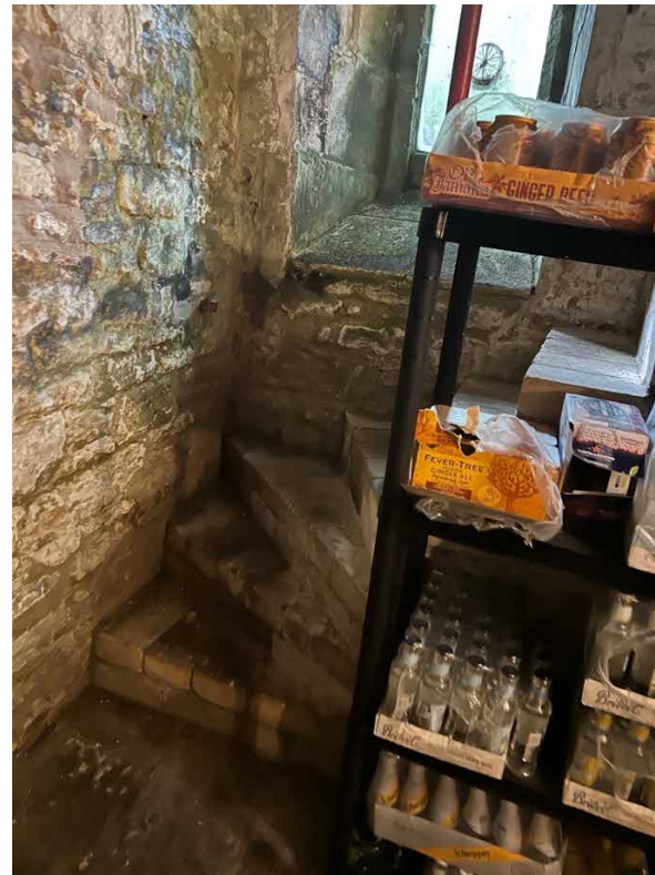
Image above: photo showing the C20 cellar stairs, albeit likely in their original position, probably lowered to ease access.
