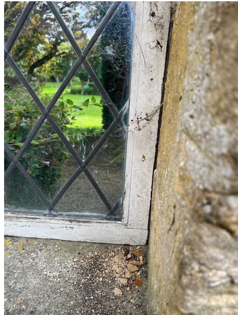
Image above: photo showing infilled opening, undertaken by Alan Mansfield Smith in the 1950s. Note the lead is clipped short and the beading is tacked on, clearly C20.
