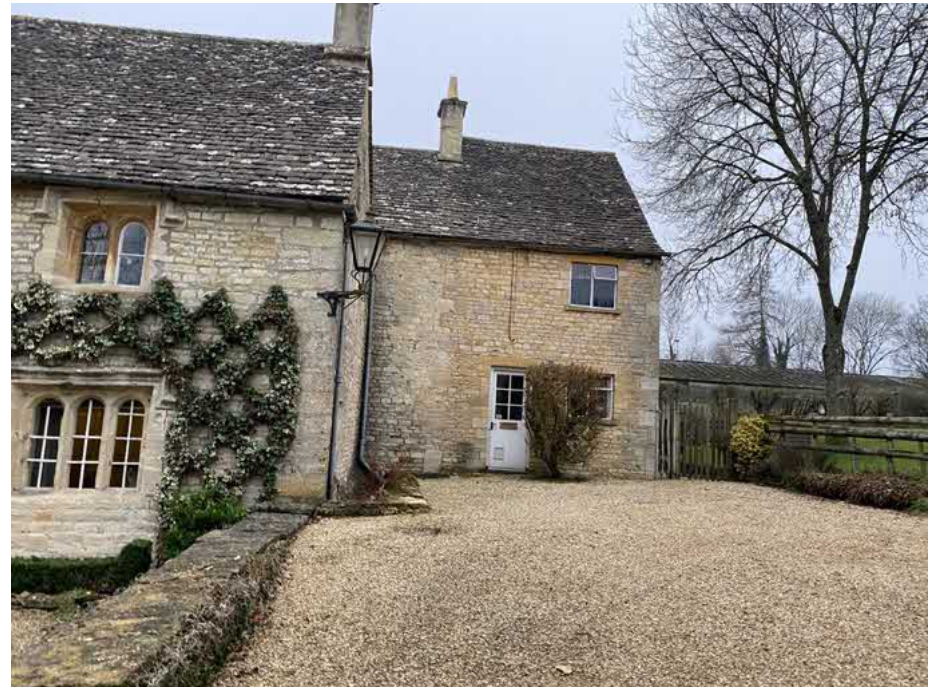
Image above: photo showing the tothing of the quoins, bleeding the earlier C19 range with the modern C20 range on the right. The C20 range might appear passable from this elevation, but the north and west flanks are constructed in Bradstone – see following sections.
