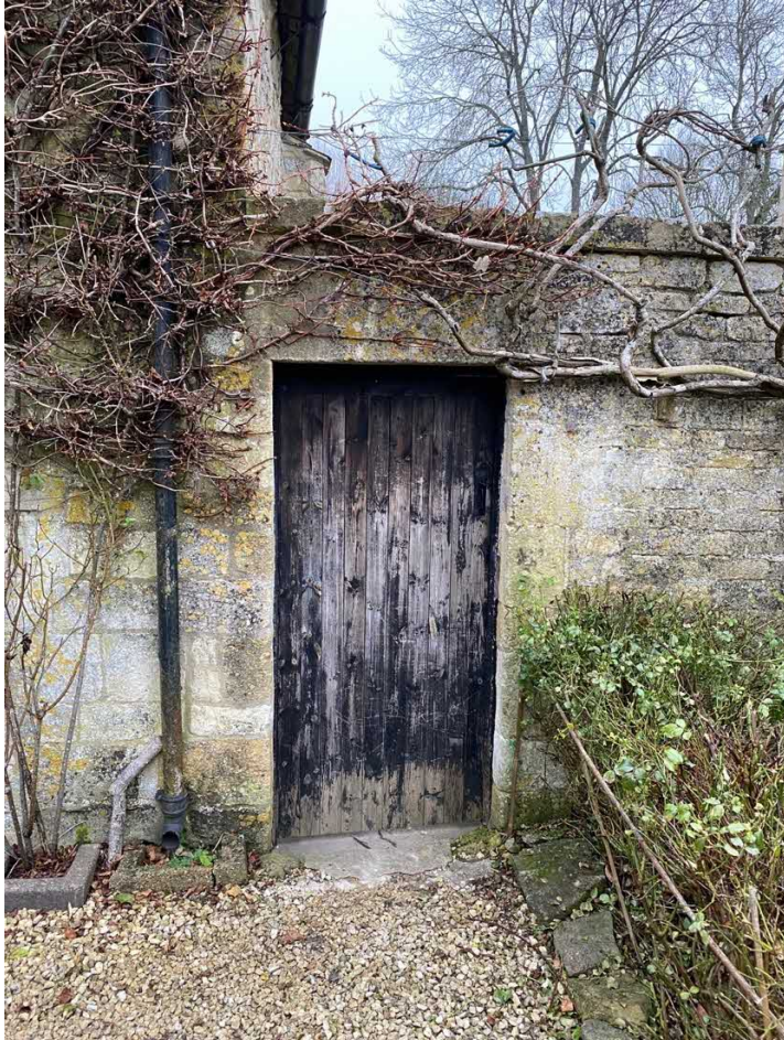
Image above: photo showing north side of third opening. This appears more historic with weathered masonry to the RHS and the Store barn gable to the LHS.
