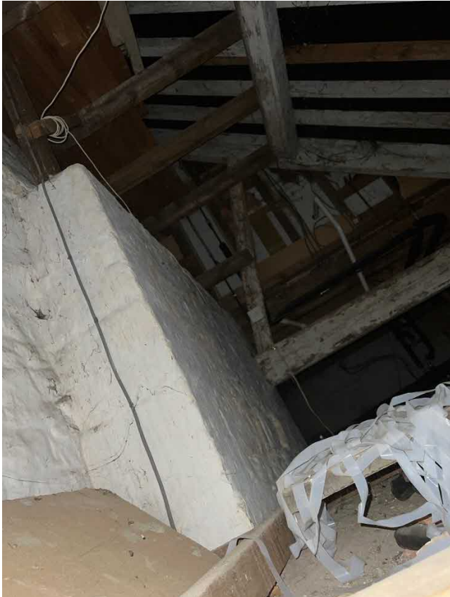
Image above showing roof void above the lean-to, where the old kitchen was located in the 1960s. Note the square purlin section and corded truss and liming of the timbers, typical of Victorian workmanship.
