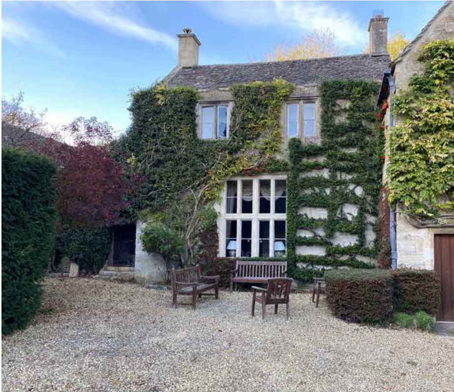
Image above: photo showing the south elevation of the early / mid C17 phase. The double height mullion window has a fine double ovolo moulding whilst the 1F window is only single. The double ovolo moulding is seen at Rectory Farm in Turkdean and is mid C17. It is thought the same mason worked on both these buildings consecutively.
