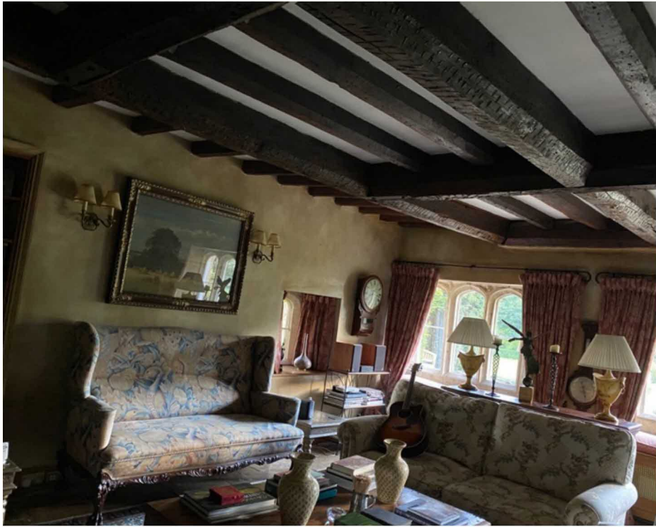
Image above: photo showing the main cruciform timber beams with the smaller section of joists on the LHS. This is likely where the stairs once existed.
