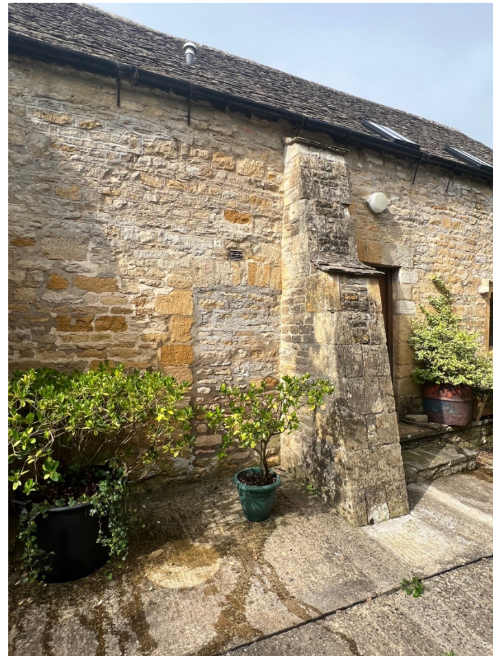
Photo showing C20 buttresses with sharp-edged quoins and cementitious mortar.
