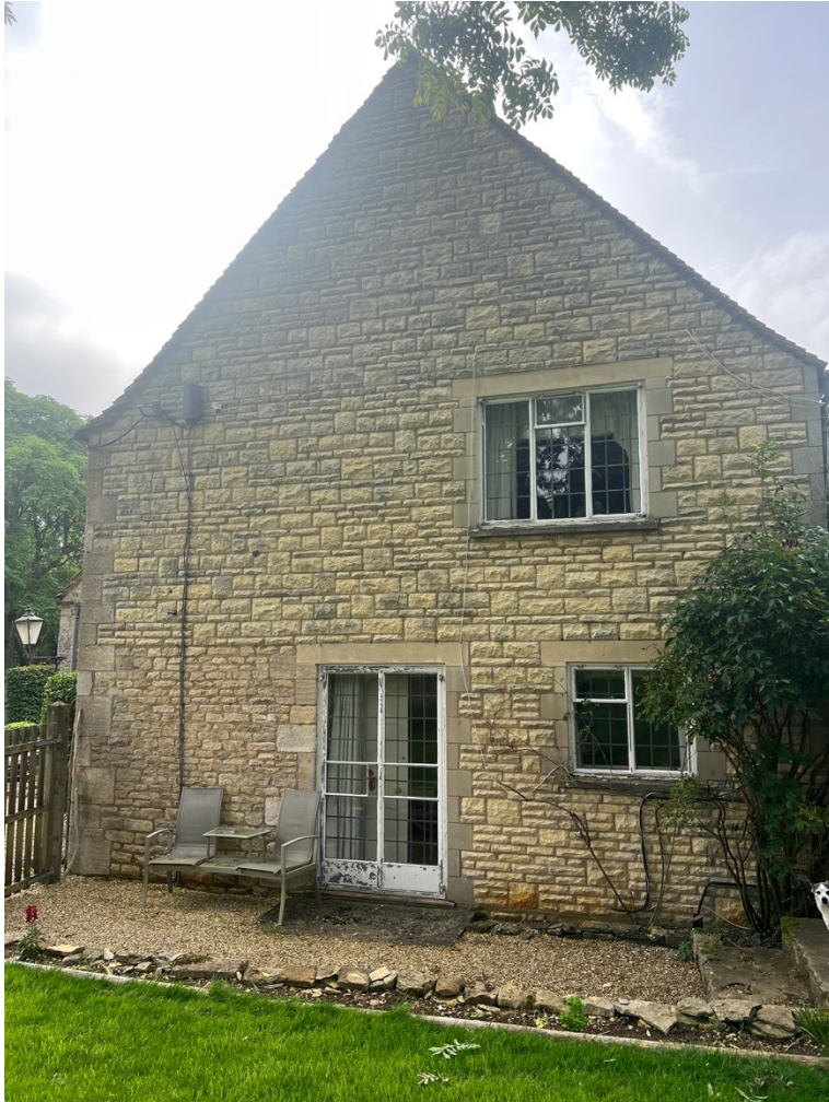
Image above showing gable end of C20 N extension. Note the use of Bradstone, albeit with a small portion of natural stone bottom LHS, likely leftovers from parts of the C19 range behind when knocked through.
