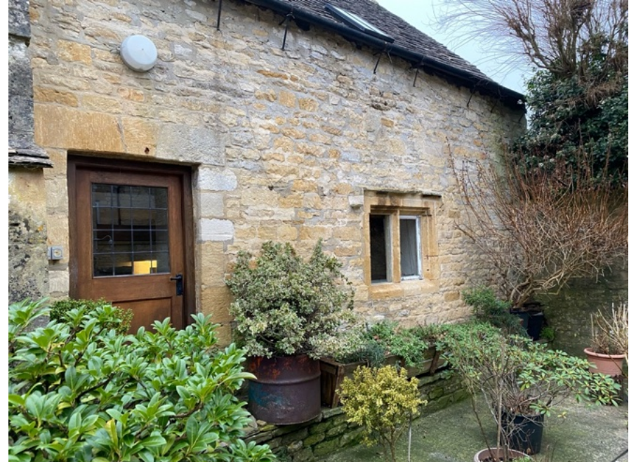
Image showing surviving mullion window. This window is to be retained and the limewash to run around its mullions, jamb and hood.
