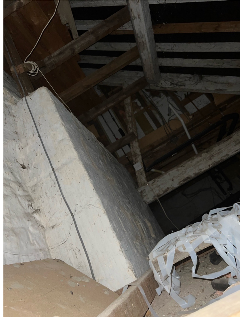
Image above showing the underside of the existing ceiling. Note the surviving truss and most of the purlin, which are to be retained. Also note the surviving rafters, which are to be re-used. The roof felt is modern, meaning the roof has been re-tiled in the C20.
