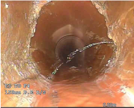
F3X_eaa49116-6e70-43e8-9044-8524c720c29c_20230907_1 15657_277.jpg, 00:00:05, 0.00 m Infiltration, running at joint at 3 o'clock, IN MH
