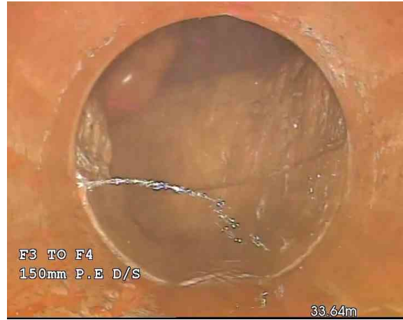
F3X_dfe36d74-ff05-4c8a-81e5-2ba0df47674a_20230907_115 940_407.jpg, 00:02:18, 33.64 m Infiltration, running at joint at 9 o'clock, IN MH
