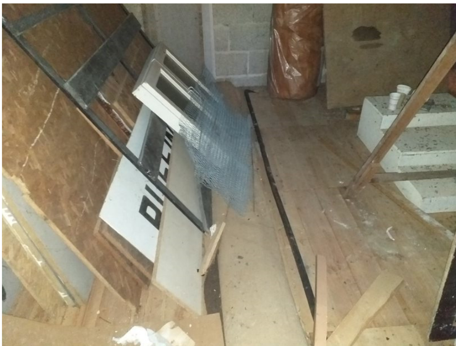
Dropping accumulations in pavilion roof void
