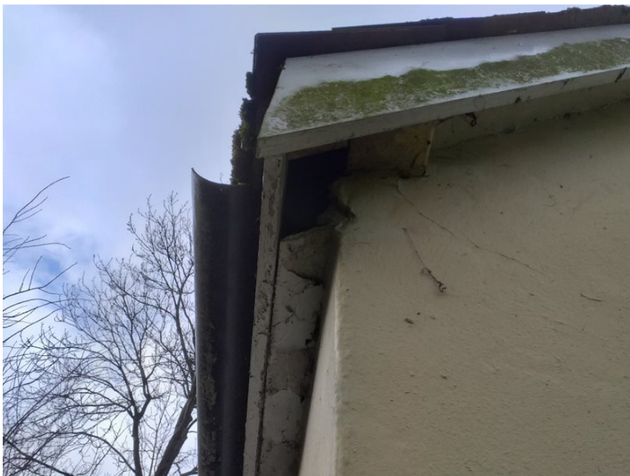
Possible bat entry/exit location on pavilion
