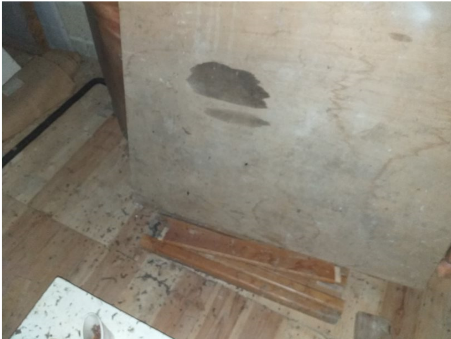
Dropping accumulations in pavilion roof void
