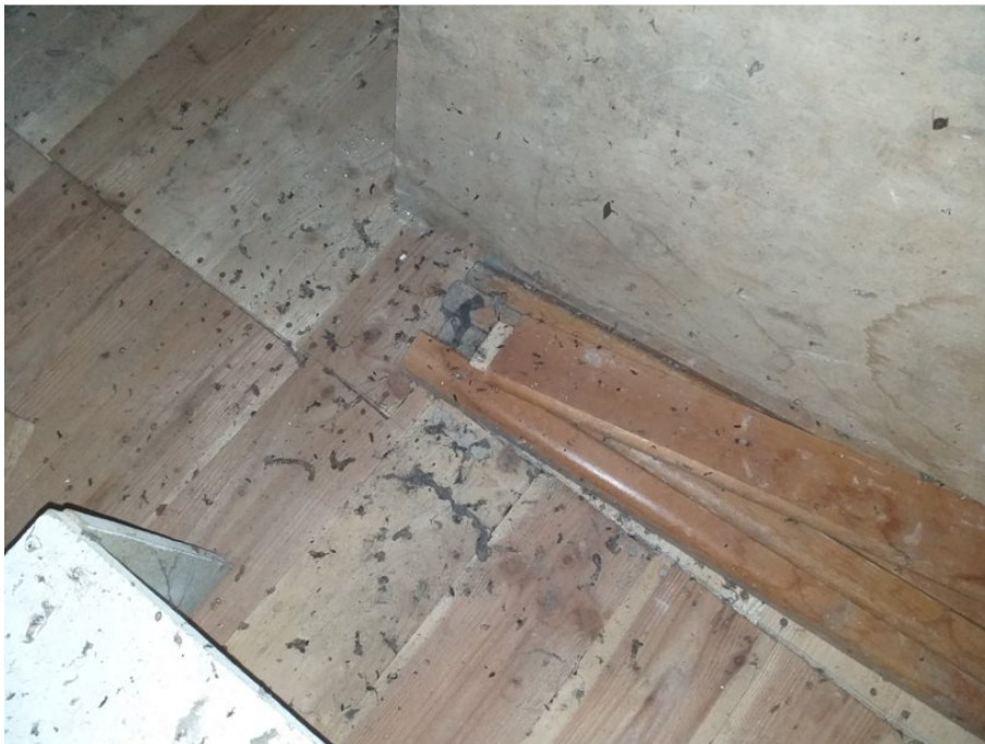
Dropping accumulations in pavilion roof void
