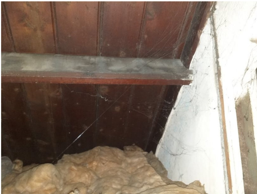
Cobwebs within void
