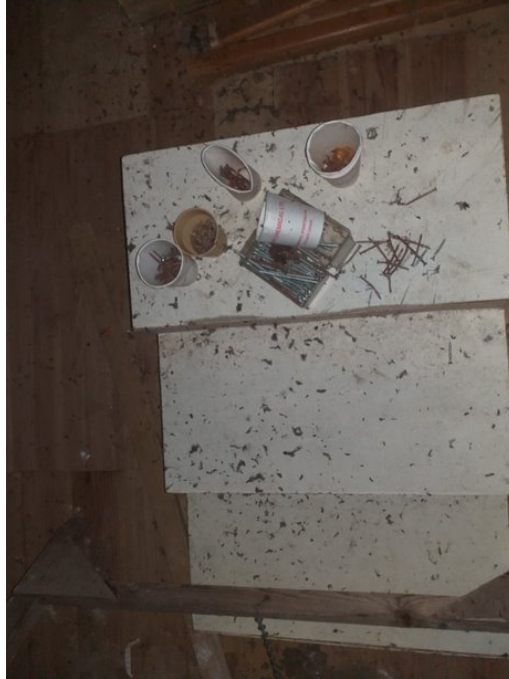
Bat dropping accumulation in pavilion roof void
