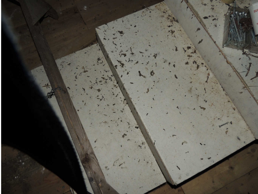
Photo 7: Bat droppings at western end of roof void
