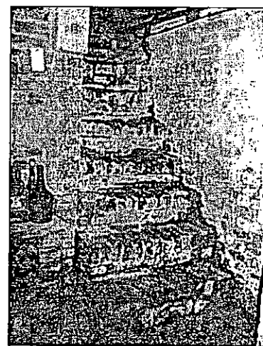
Figure 17: Cellar, brick steps in southwest corner leading up to the lounge (room 3)
