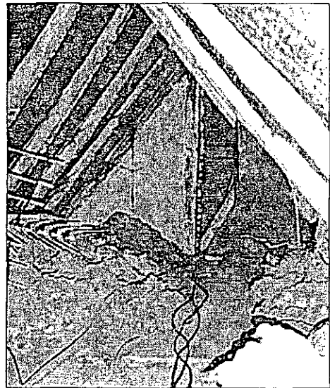
Figure 55: Southern end of roof space. Timber rafters and the lath and plaster partition are visible
