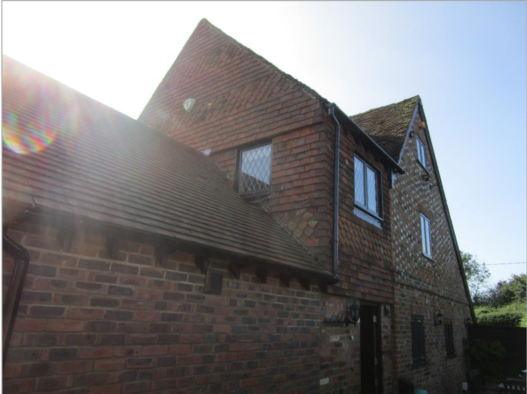
Fig. 5: The roof of the 2010 kitchen addition awkwardly abuts the first floor window of the 1991 addition.
