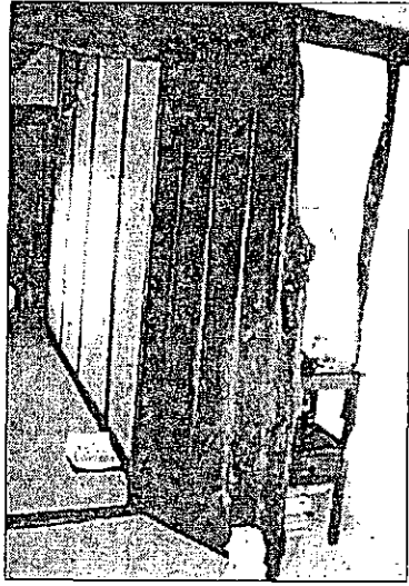
Figure 50: Room 15. Timber tongue and groove board doorway at west end of north elevation (early nineteenth century)
