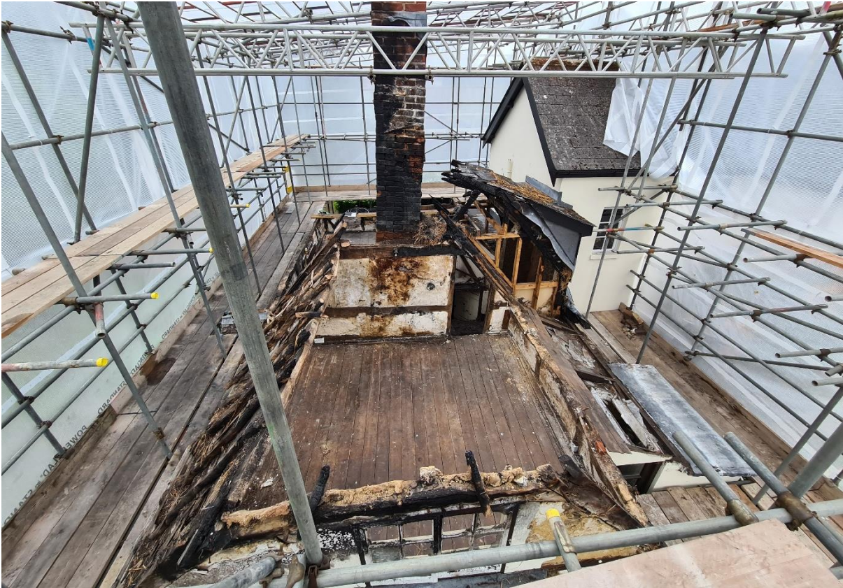
View from above showing extent of fire damage to frame.
