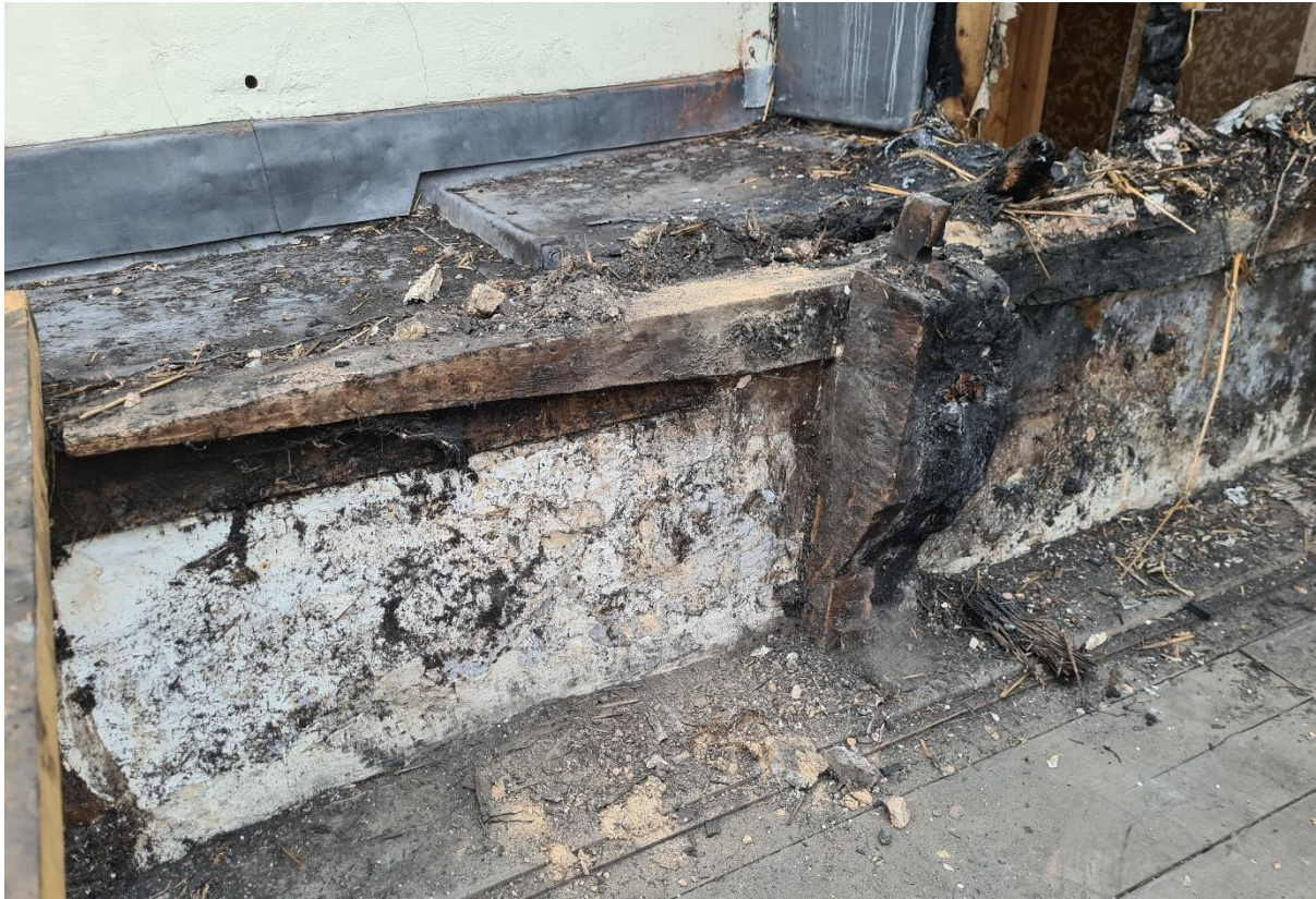
Jowl post in north wall – note teazle tenon remnants, suggesting there was originally a tie beam here. Also note the patch repair to the wall plate – removing any evidence of a lap-dovetail joint for the tie beam.
