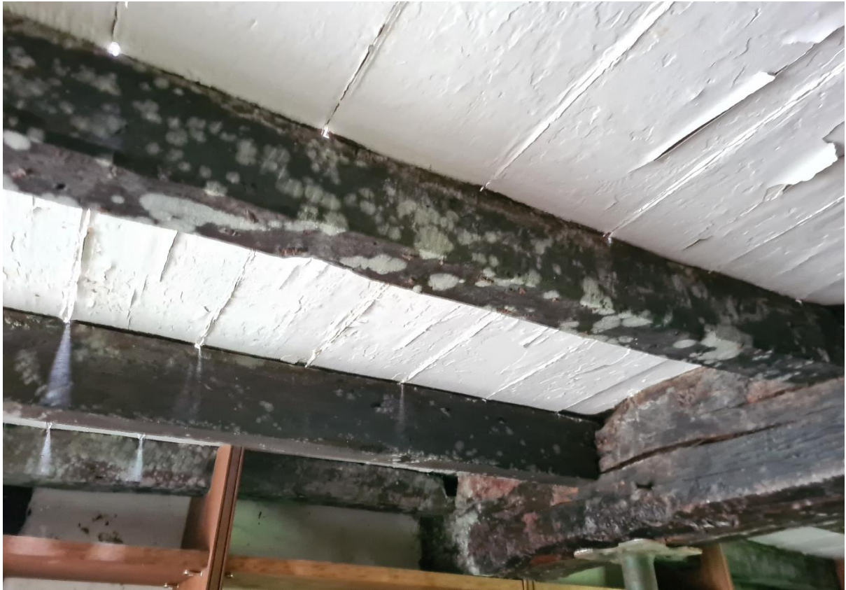
Mould is flourishing on the floor framing due to the rise in moisture levels putting out the fire. It is particularly worse on components with a higher sapwood content making them very much more susceptible to further decay.
