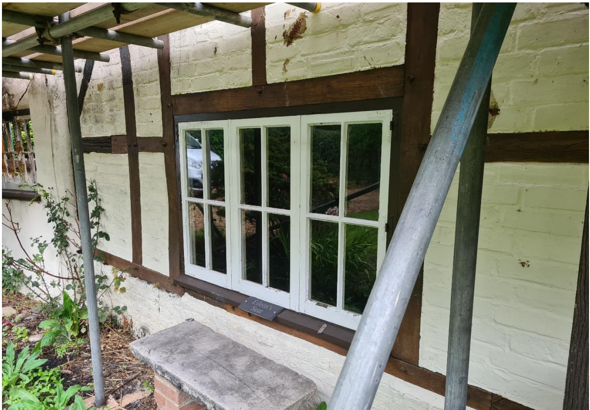
Exterior view at southwest corner of frame. This area of framing has been rebuilt to a good standard, although historically there would have been a jowled storey post in the middle of the window. I suspect that the current window replaces a Victorian window which cut through the post making restoration of the post seem pointless to previous occupants.
