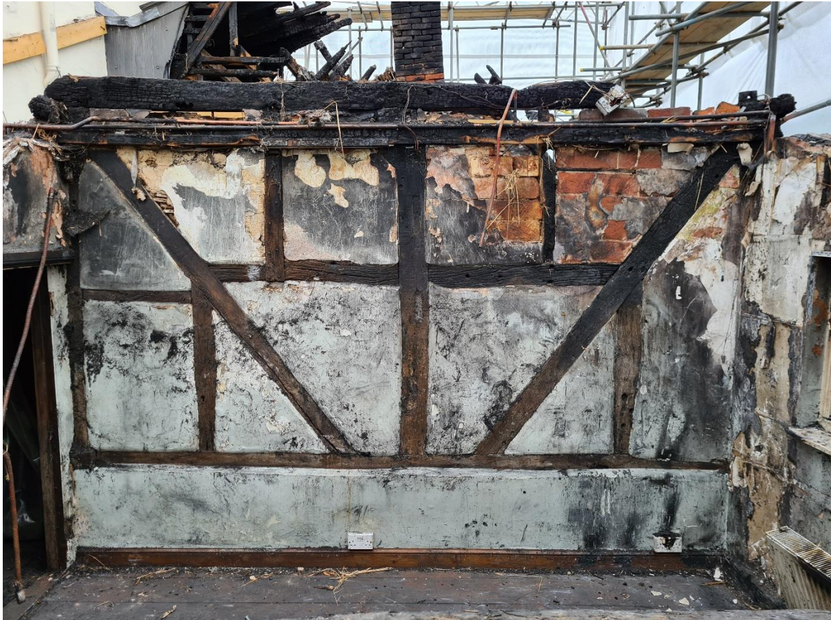
West gable – note tie beam – it will need to be scarfed for just over half it's length as well as an external face patch.
