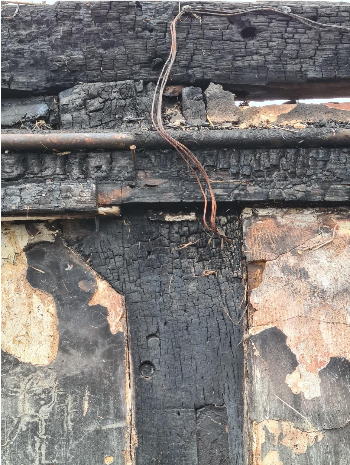
Jowl post re-used within west gable. Note tenon for wall plate (at top, to the right of cabling) proving it was used elsewhere prior to this frame, also void mortices below. The peg within the gable tie beam is NOT associated with this connection – there is no tenon there.
