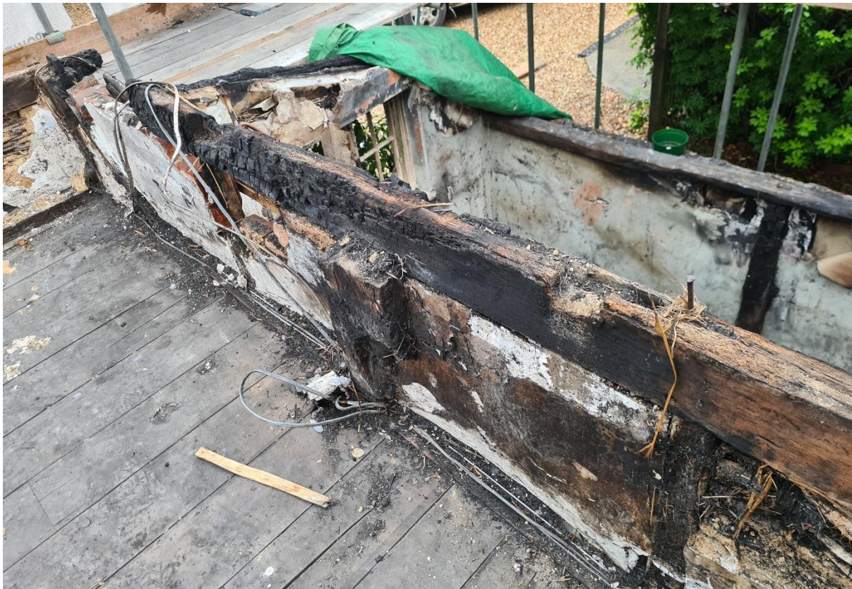
Internal view of west gable tie beam. From just to the right of the central post it is basically sound, albeit scorched.
