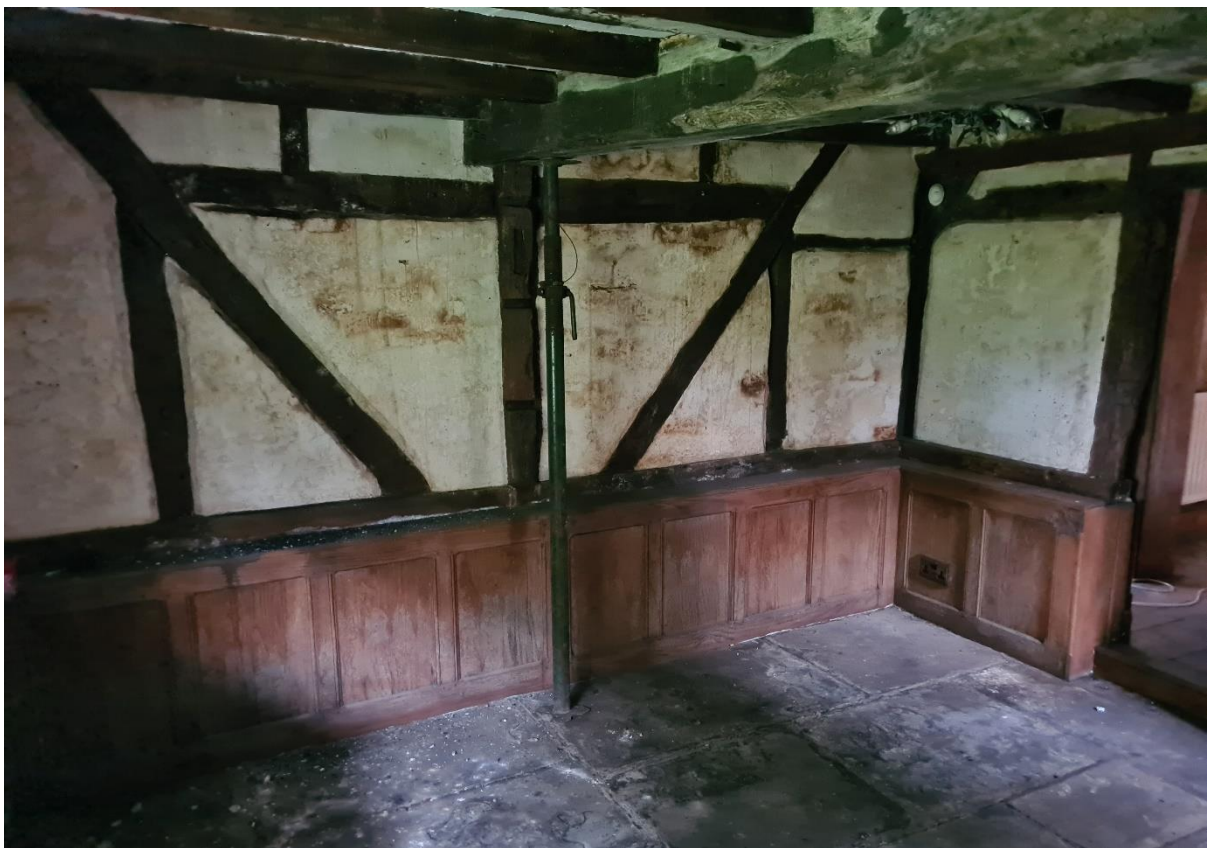
Interior of ground floor room, west end. Note low-level paneling – this should be opened up to check the moisture content and condition of sole plate and bottoms of studs/posts. This will also allow air flow to the area and speed up drying out of the building fabric.
