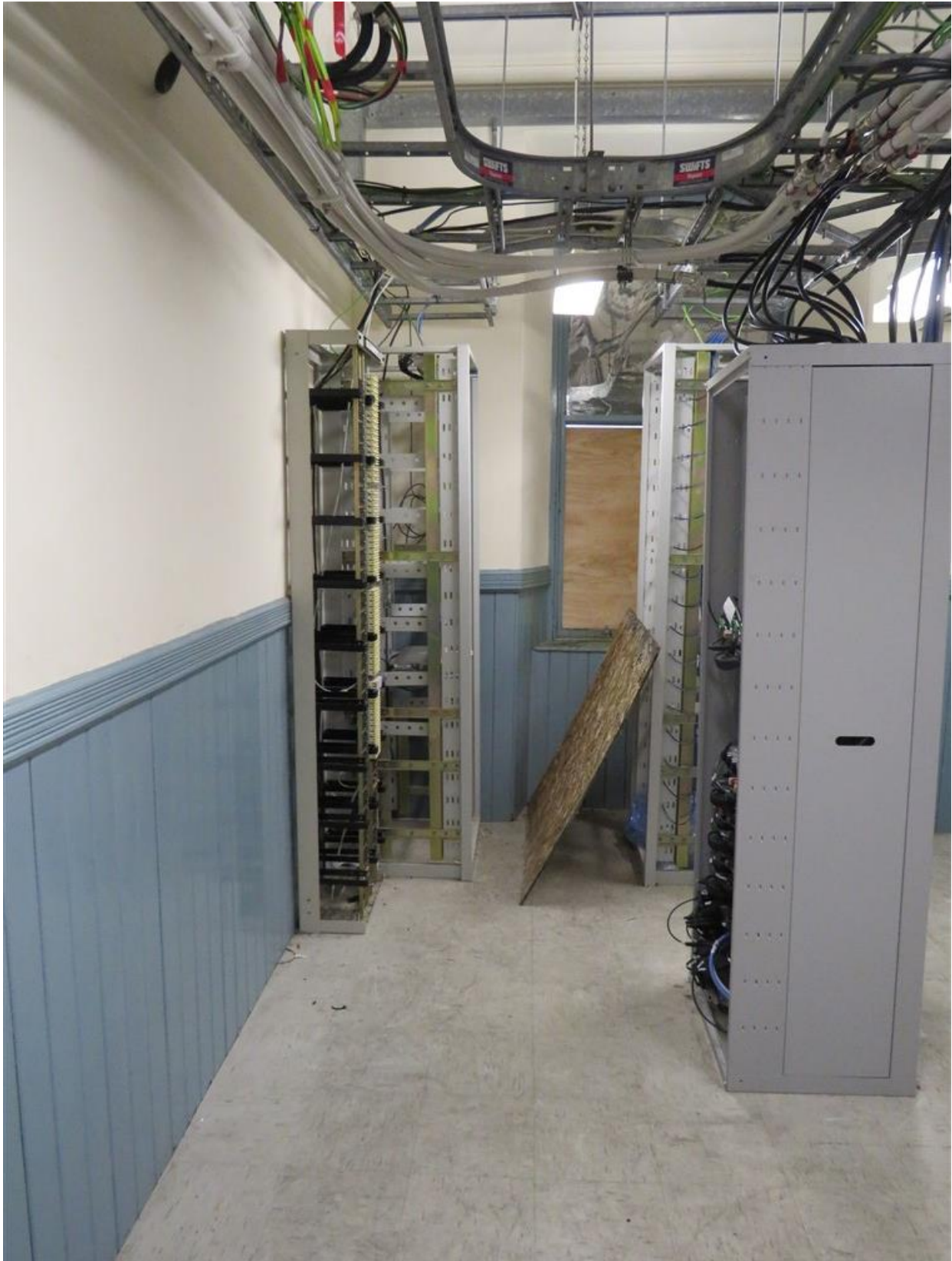
Photograph 2: Existing Equipment Room
