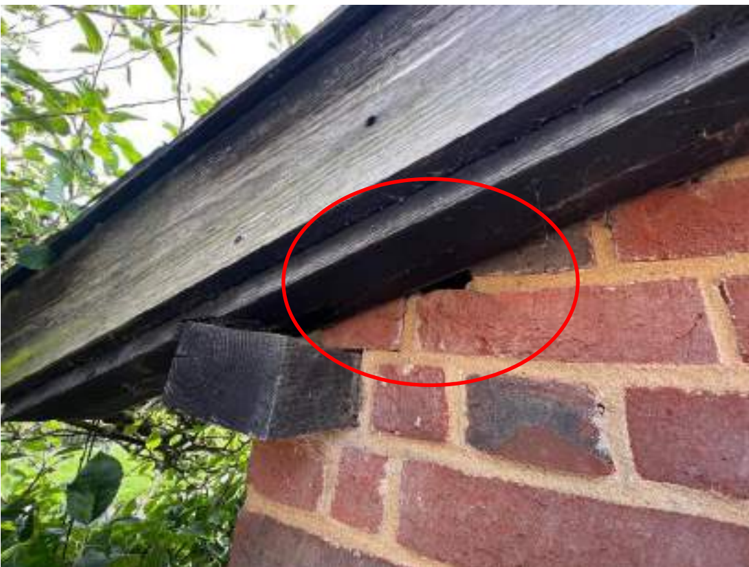
Photo 10. Close up of building 6, electrical unit. Shows gap between brickwork and timber as shown by red circle. Photograph taken on 23 September 2023.
