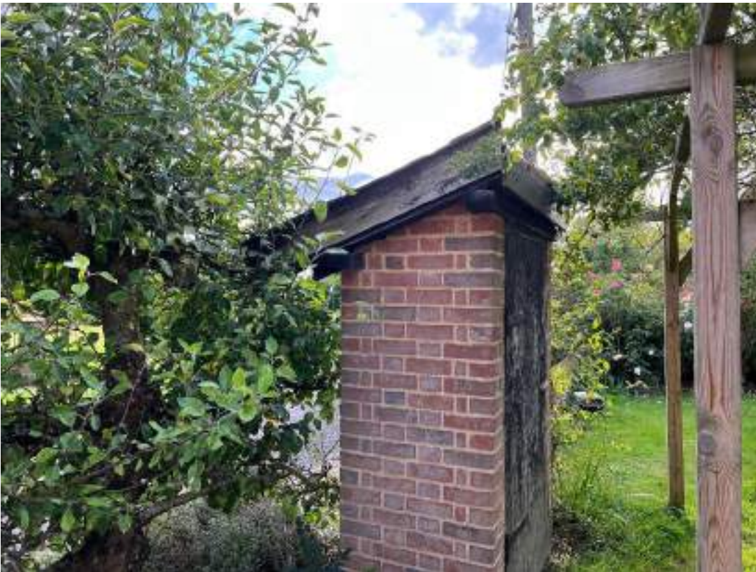
Photo 9. View of building 6, electrical unit. Photograph taken on 23 September 2023.
