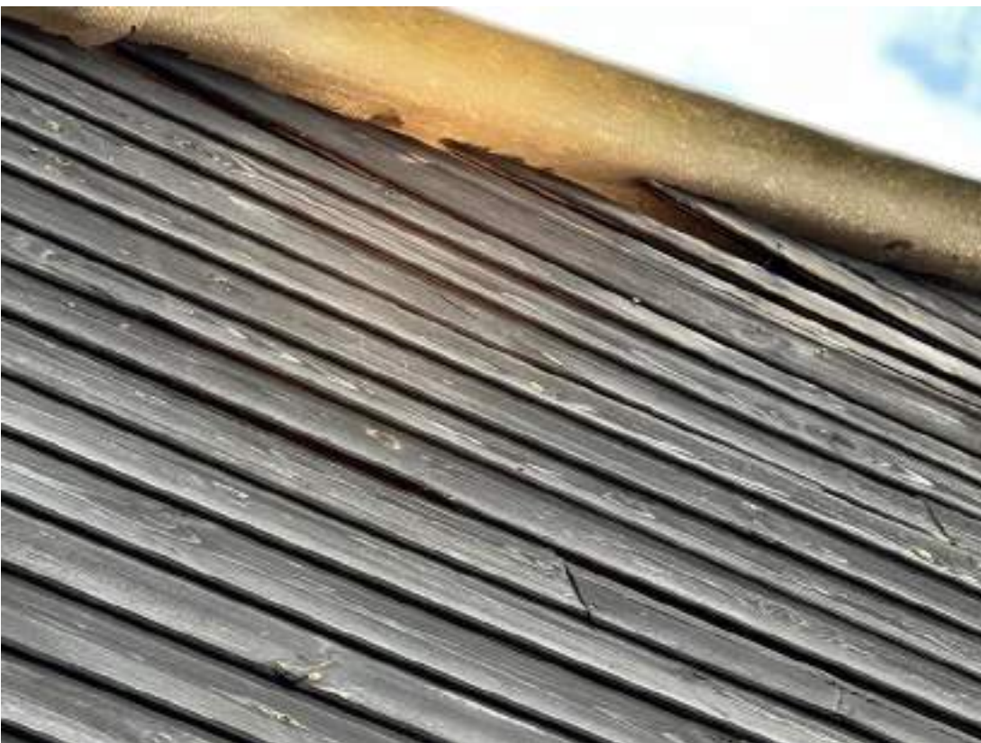
Photo 16. View of south gable of building 3. Shows lifted cladding and gaps under roofing material. Photograph taken on 23 September 2023.
