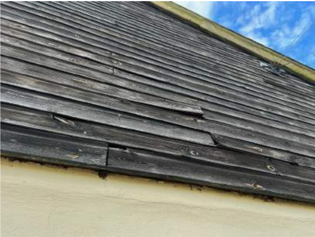
Photo 14. View of south gable of building 3. Shows lifted cladding. Photograph taken on 23 September 2023.
