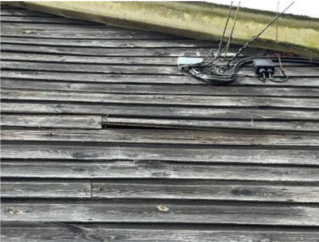
Photo 15. View of south gable of building 3. Shows lifted cladding. Photograph taken on 23 September 2023.
