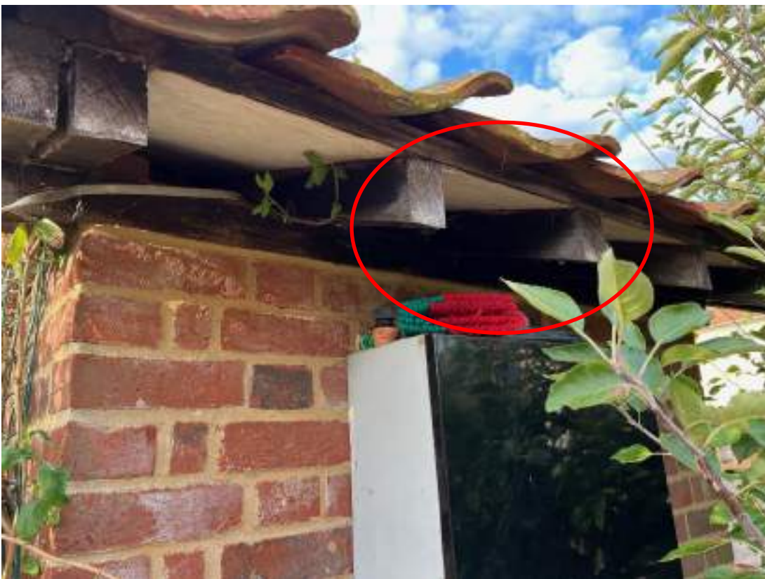
Photo 12. Close up of building 6, electrical unit. Shows gap under eaves as shown by red circle. Photograph taken on 23 September 2023.
