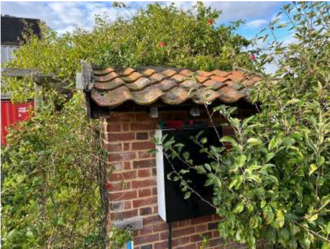
Photo 11. Close up of building 6, electrical unit. Photograph taken on 23 September 2023.
