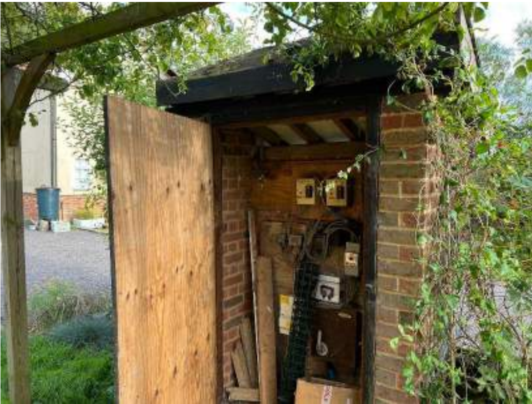
Photo 13. Internal view of building 6, electrical unit. Photograph taken on 23 September 2023.
