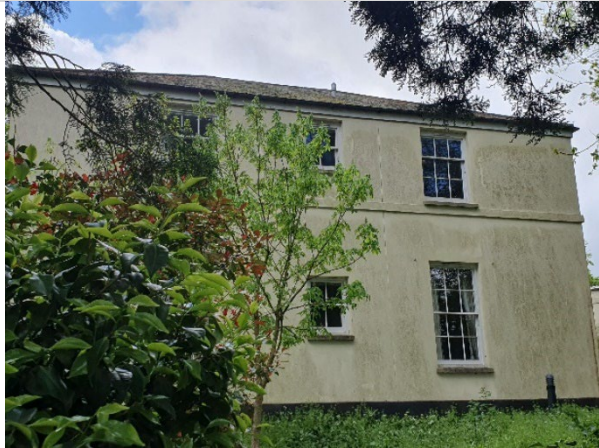
External features – bargeboard – lifted – south aspect
