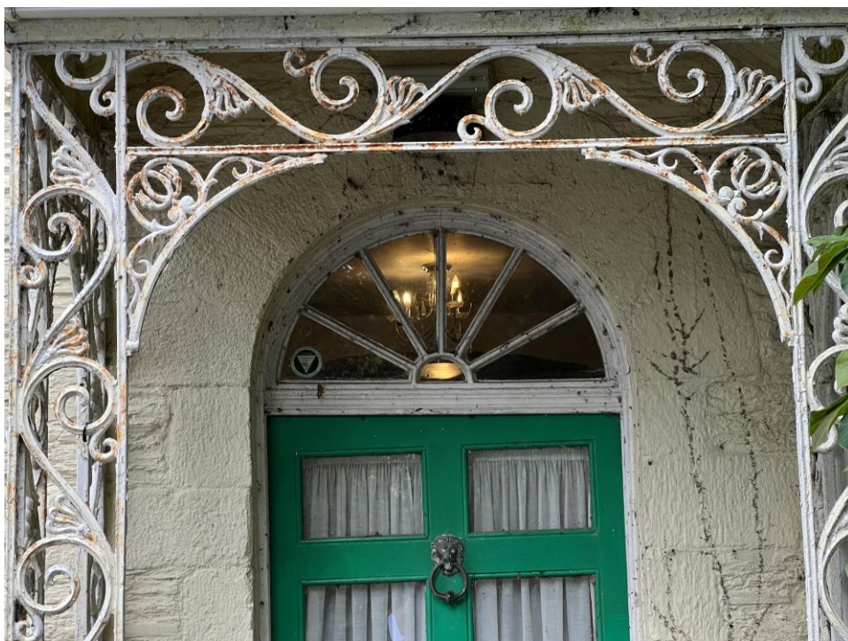
Fig 10 Distortion in doorway to west elevation.
