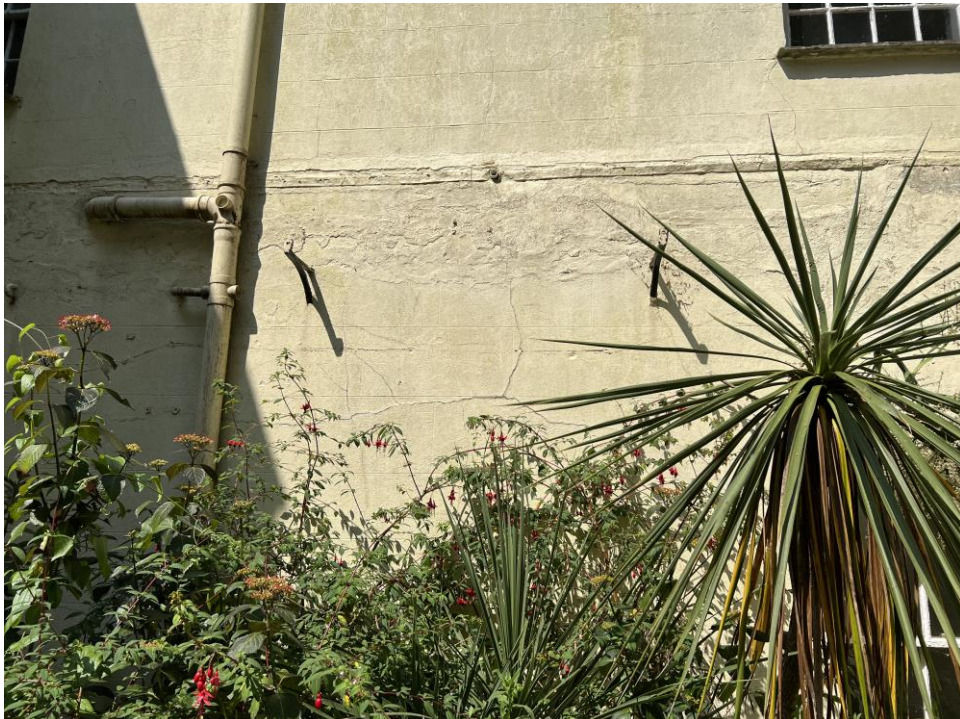
Fig 7 Cracking to east elevation of original building
