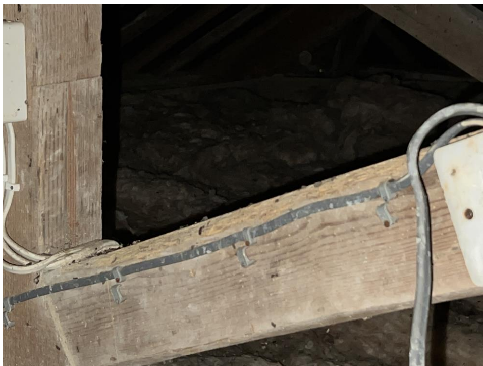
Fig 18 Wood-boring beetle attack to truss member adjacent to roof hatch.
