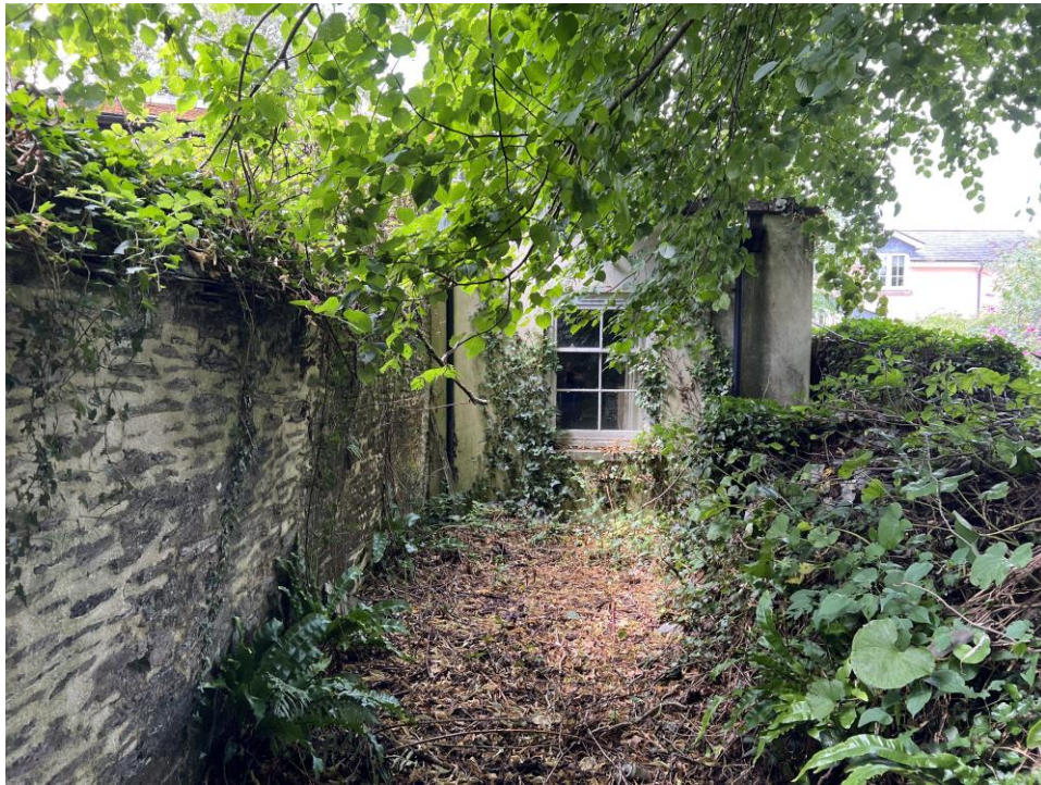
Fig 11 External garden wall and intersection with single storey building to north of house.
