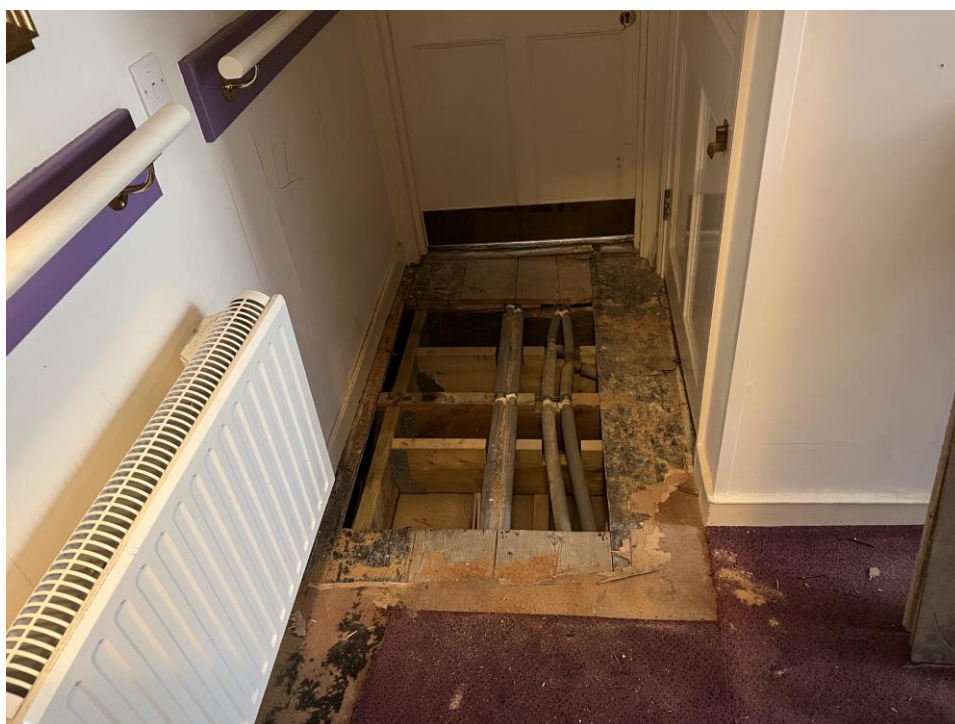
Fig 14 Trimmed first floor joists in location 4
