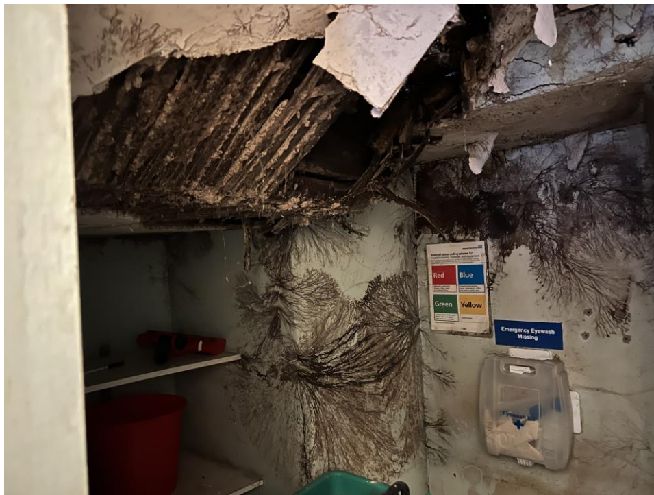
Fig 13 Dry rot under main staircase in original building.
