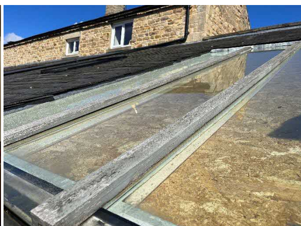
External outer panes of glazing
