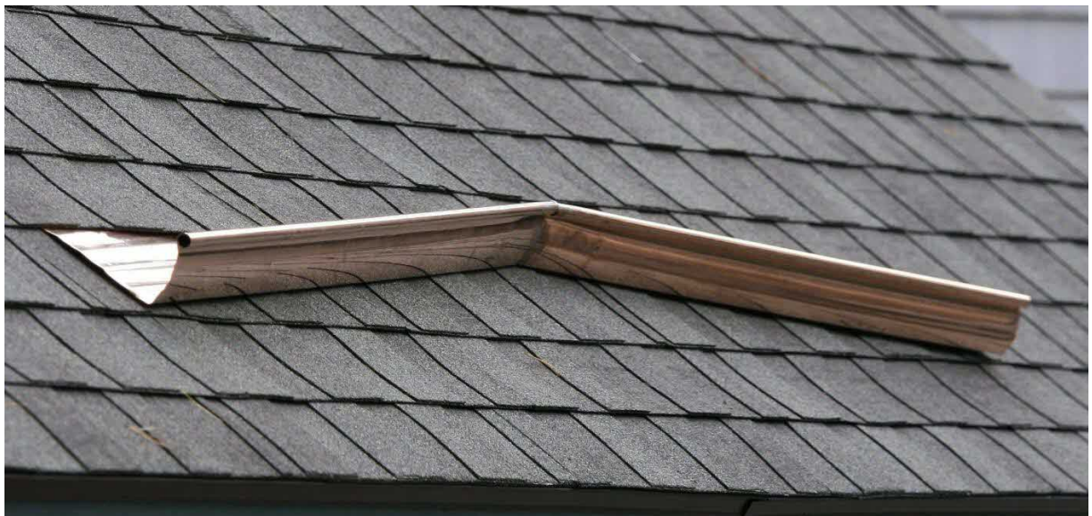
Roof flow diverter
