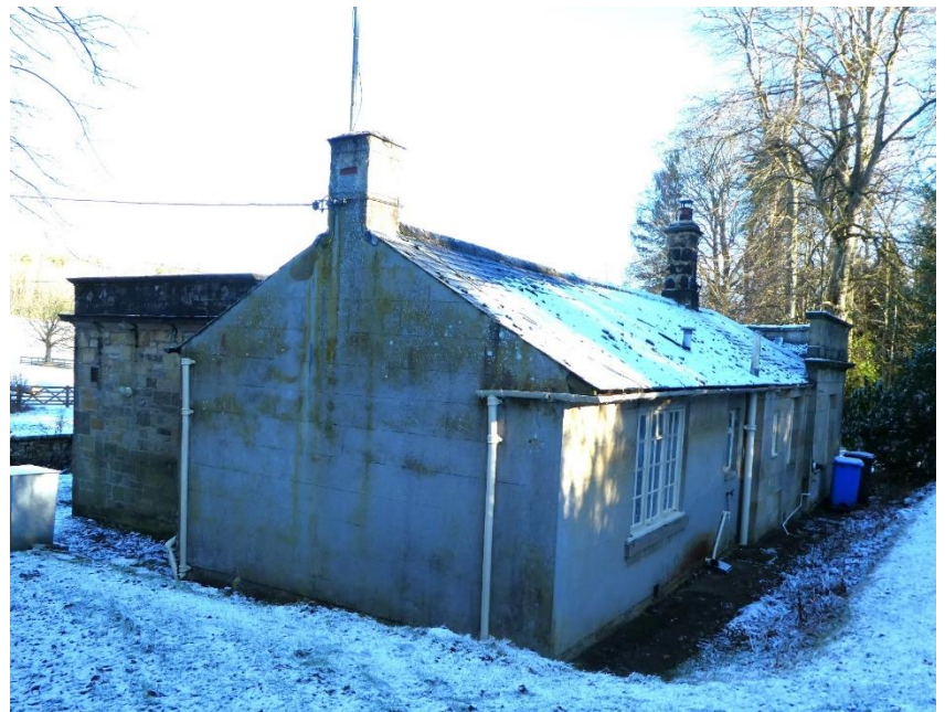
WEST ELEVATION, from South West. Existing Kitchen to left, existing Bedroom to right, all part of the later extension.
