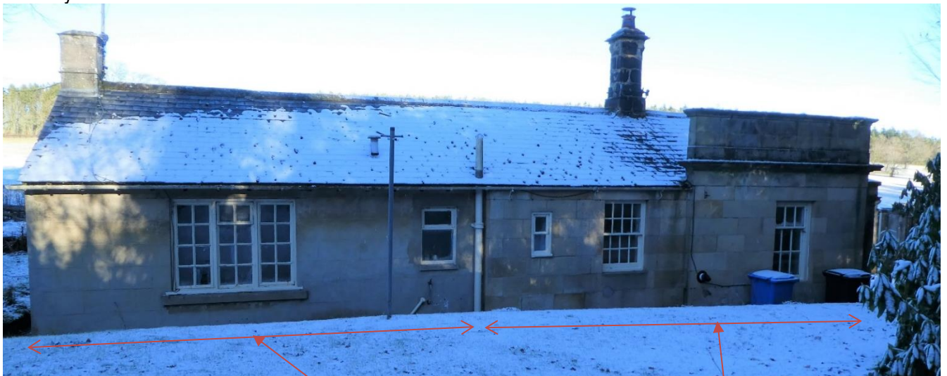
SOUTH ELEVATION. Existing Bedroom and Bathroom, all part of the Later Extension. Bedroom 2, Liv Room: the original building
