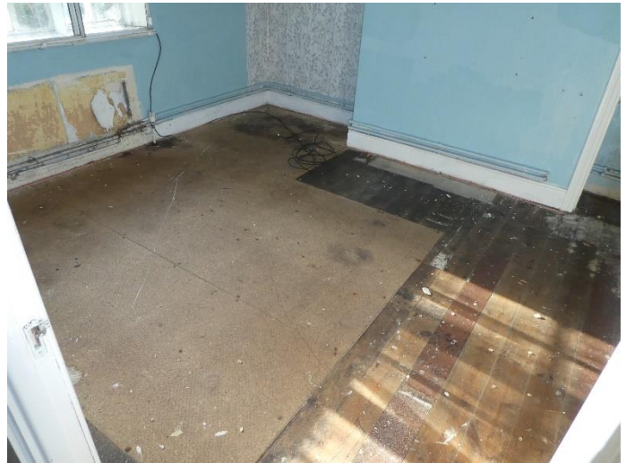
Floor, - previous repairs in particle board
