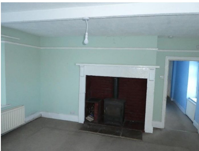
Liv Room fireplace – prior to ceiling collapse
