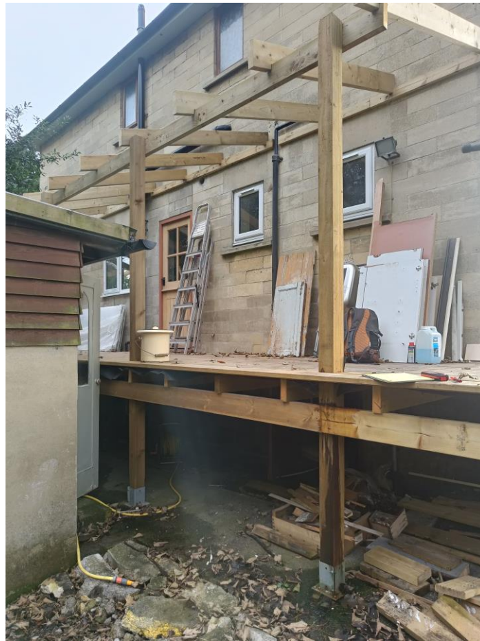
Image 3: the construction of the decking on the north-east elevation of the dwelling showing the timber posts bolted to the pre-existing concrete path.
