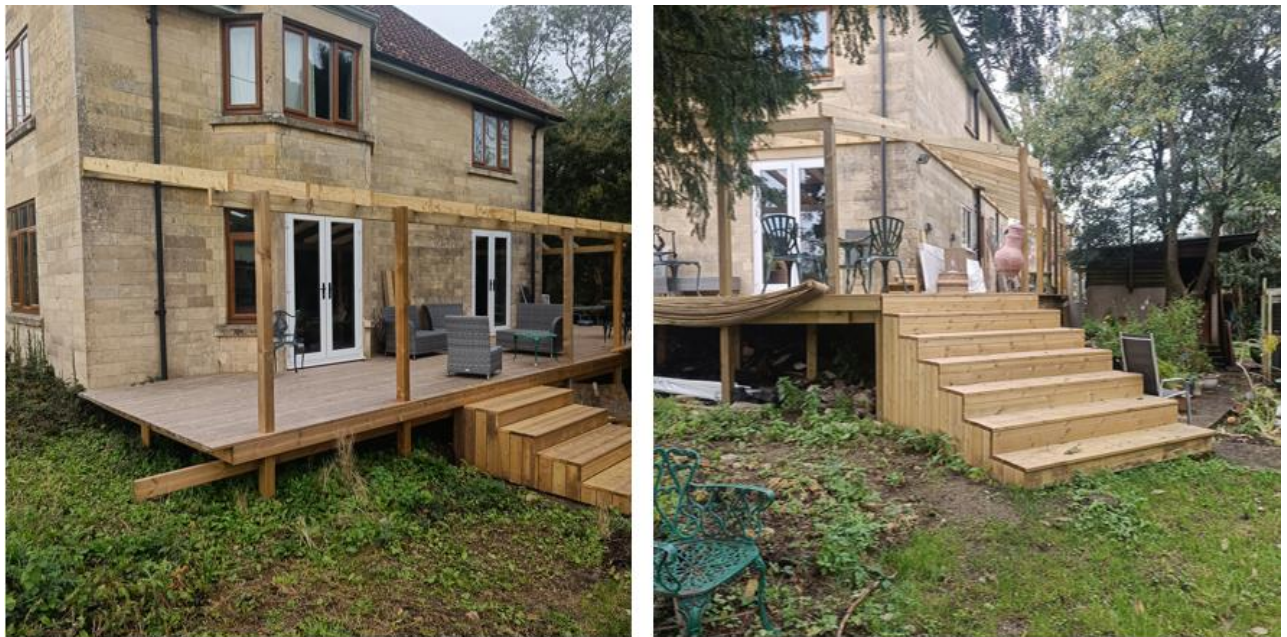
Image 1 and 2: the decking and pergola structure that has been completed to date.
