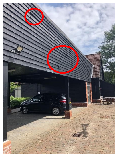
Figure 1: Warped timber cladding on Build B1
