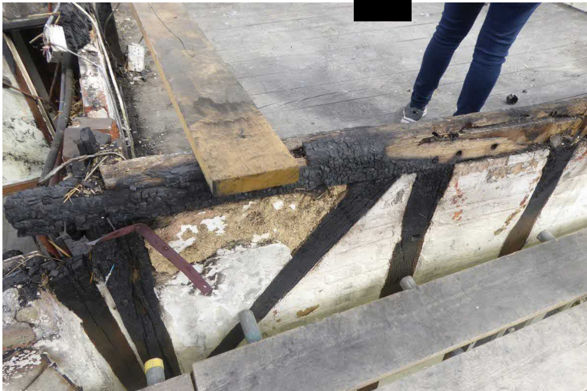
Figure 1: Surviving panels of wattle and daub- first floor, south elevation
