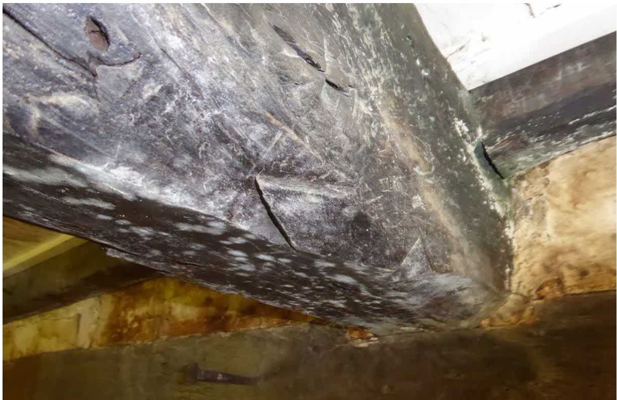
Figure 10: Chamfered stop to spine beam, Room G1 – early 17 th century
