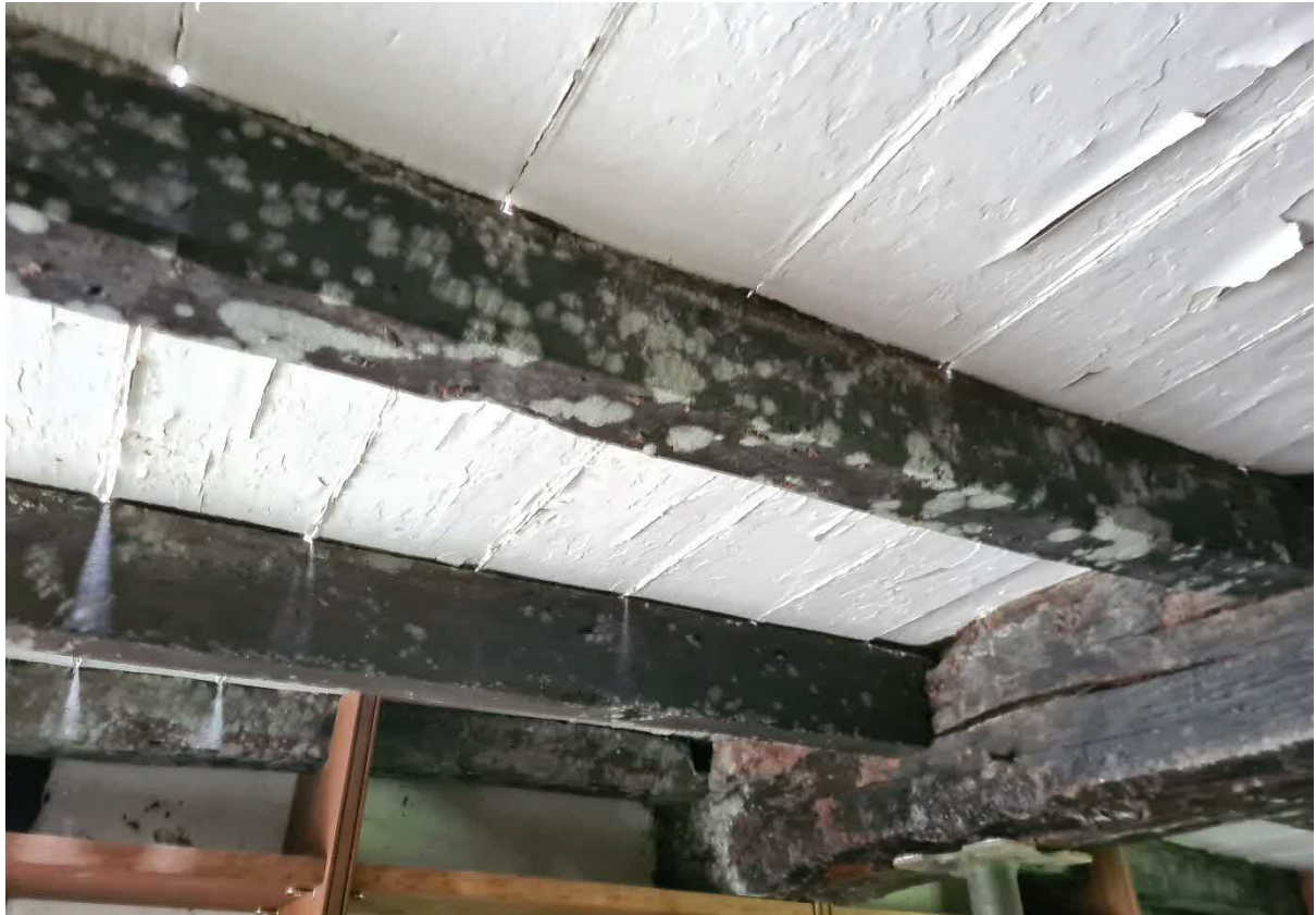
Mould is flourishing on the floor framing due to the rise in moisture levels putting out the fire. It is particularly worse on components with a higher sapwood content making them very much more susceptible to further decay.
