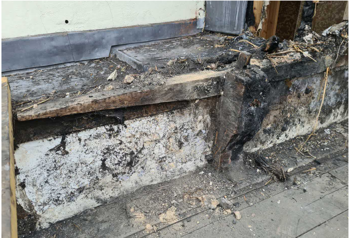
Jowl post in north wall – note teazle tenon remnants, suggesting there was originally a tie beam here. Also note the patch repair to the wall plate – removing any evidence of a lap-dovetail joint for the tie beam.
