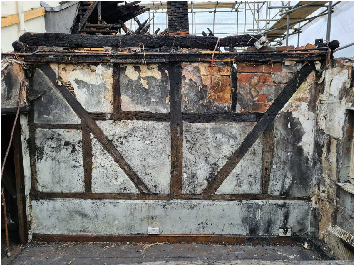
West gable – note tie beam – it will need to be scarfed for just over half it's length as well as an external face patch.
