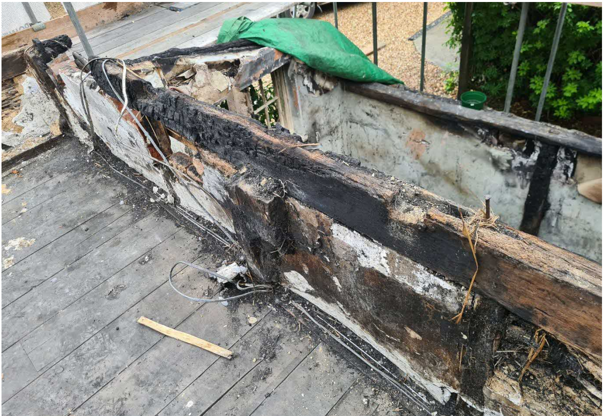
Internal view of west gable tie beam. From just to the right of the central post it is basically sound, albeit scorched.
