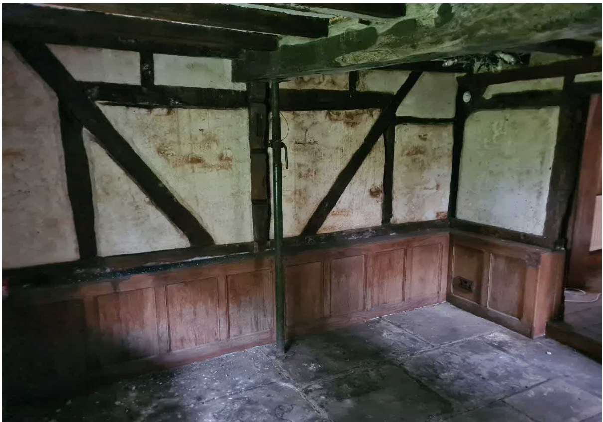
Interior of ground floor room, west end. Note low-level paneling – this should be opened up to check the moisture content and condition of sole plate and bottoms of studs/posts. This will also allow air flow to the area and speed up drying out of the building fabric.
