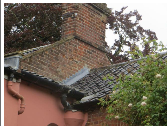
Roofing area where the service wing adjoins the main property and 'lean-to'. Pantiles.
