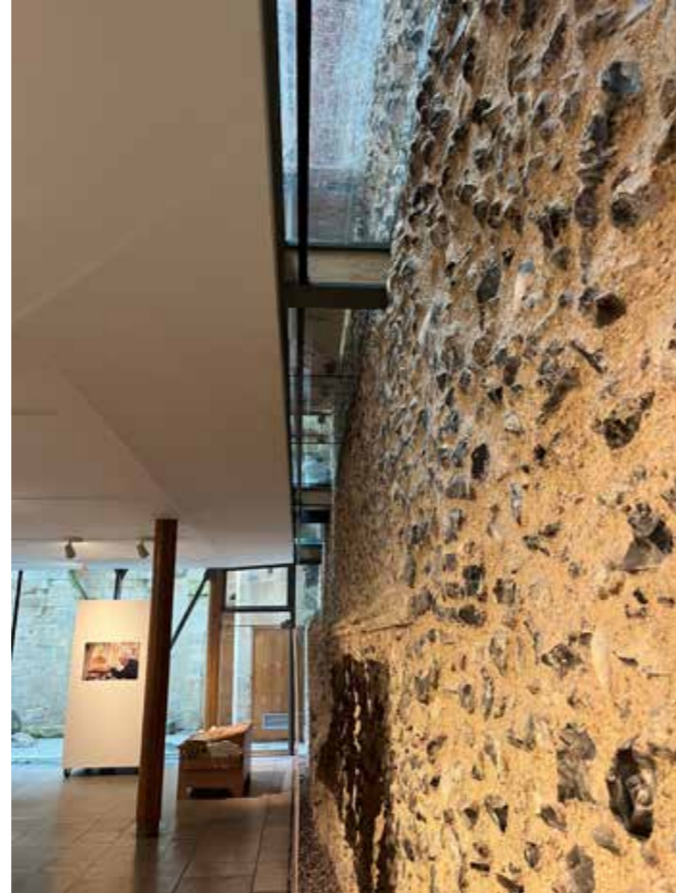
Precedent image; Hopkins Architects utilised glazed abutments at grade I Norwich Cathedral to express the separation between new Hostry and old building fabric.
