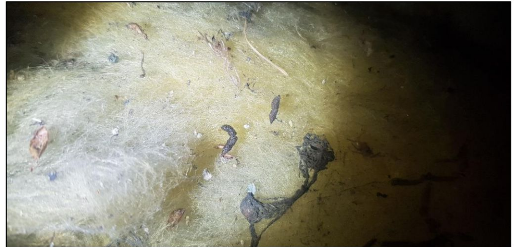
Picture 4: Bat droppings found near northern gable end of loft space.
