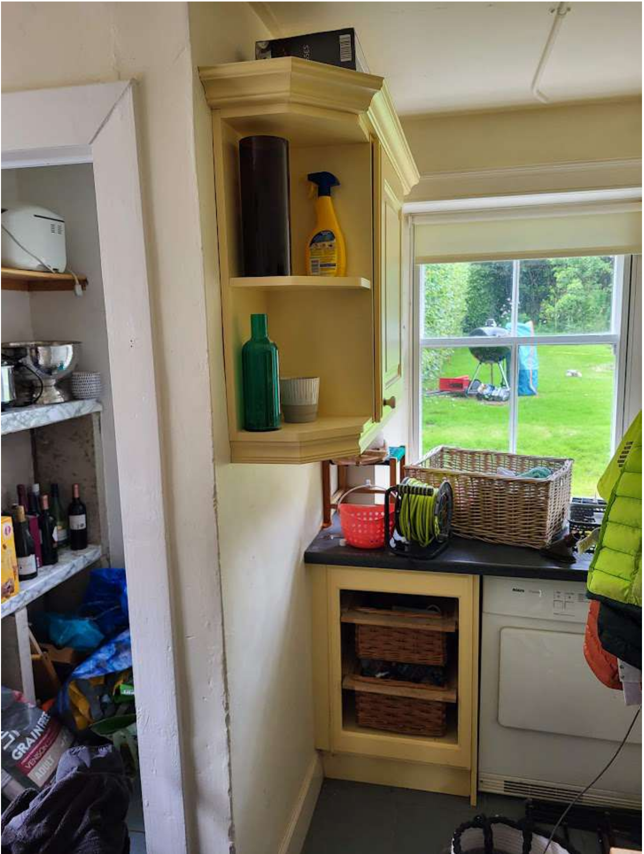
PHOTO OF THE EXISTING UTILITY ROOM WINDOW FROM THE INSIDE WHICH IS PROPOSED TO BE A DOOR OUT TO THE GARDEN.
