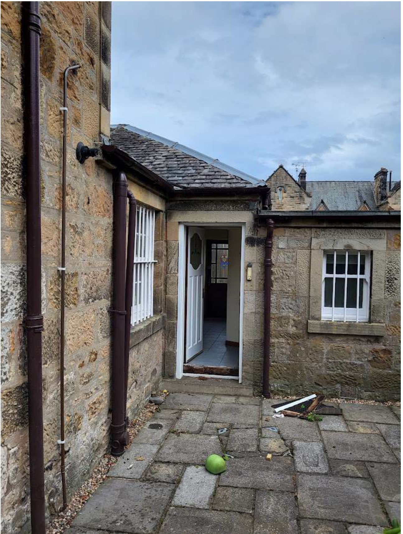
THE EXISTING COURTYARD SHOWING THE EXISTING KITCHEN WINDOW AND WC WINDOWS WITH BARS
