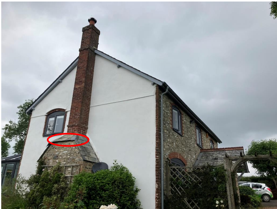
Plate 5 - Uplifted lead flashing/roof tile at the base of the chimney on the southern elevation
