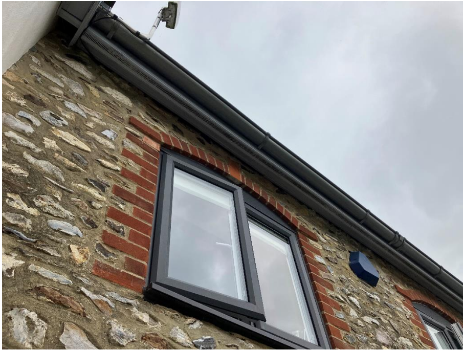
Plate 4 - Wall top access into the loft space on the western elevation of the house
