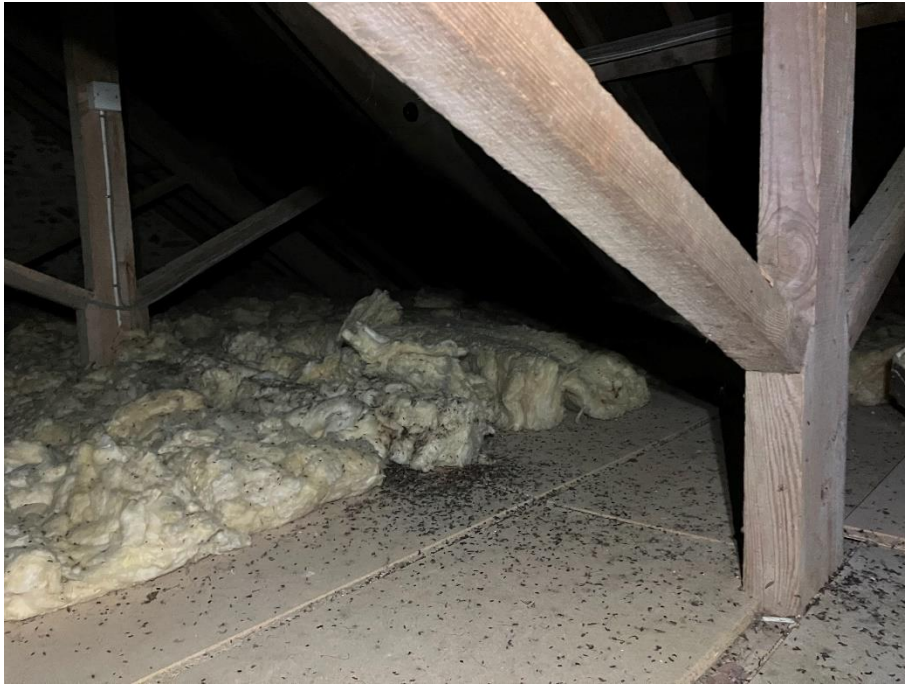
Plate 8 - Long-eared droppings in the loft space both under the ridge and scattered on the insulation
