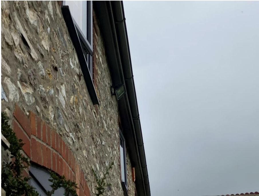
Plate 6 - Wall top access into to the loft space on the eastern elevation
