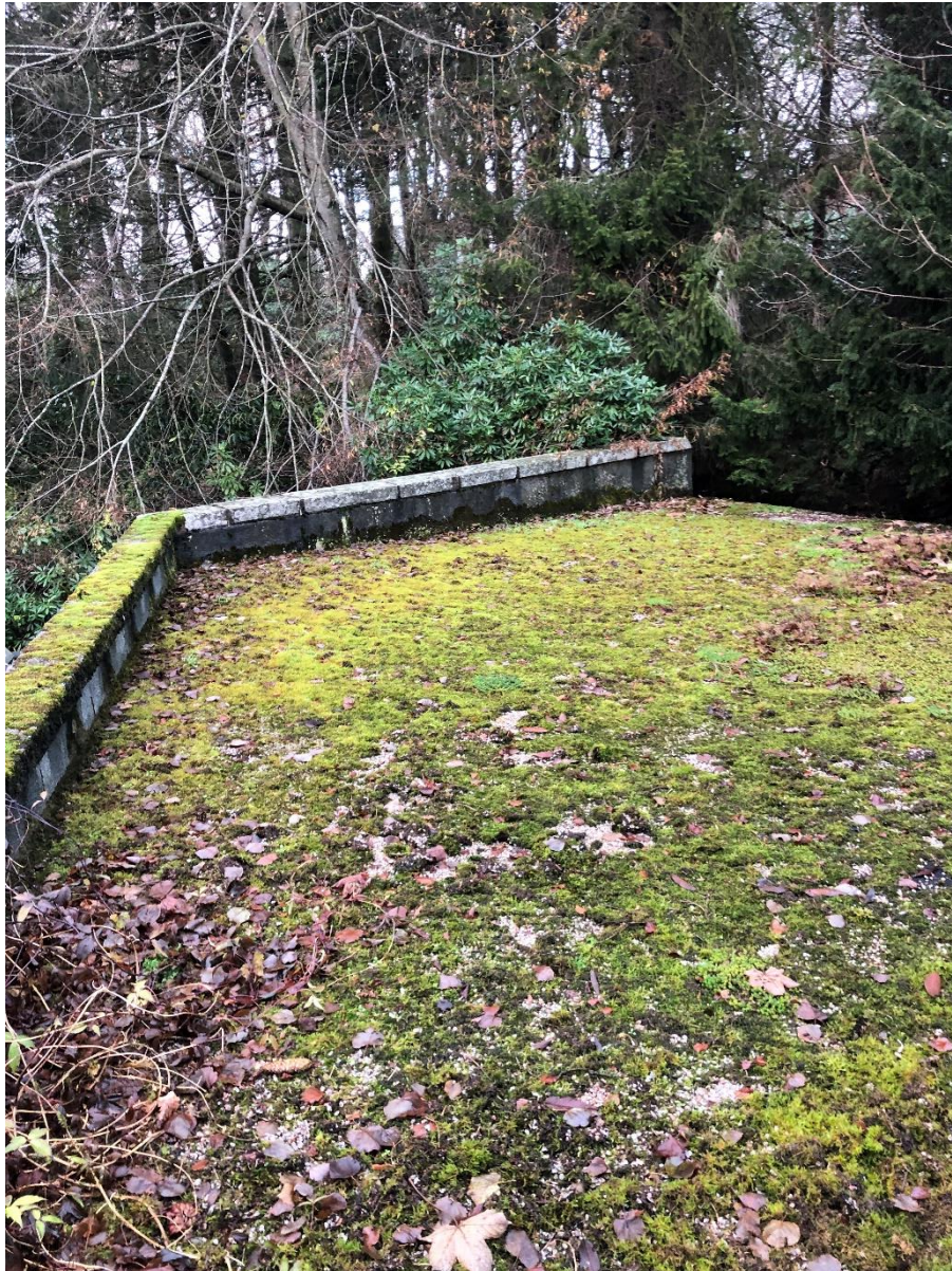
The roof of the extension is currently overgrown with biological materials
