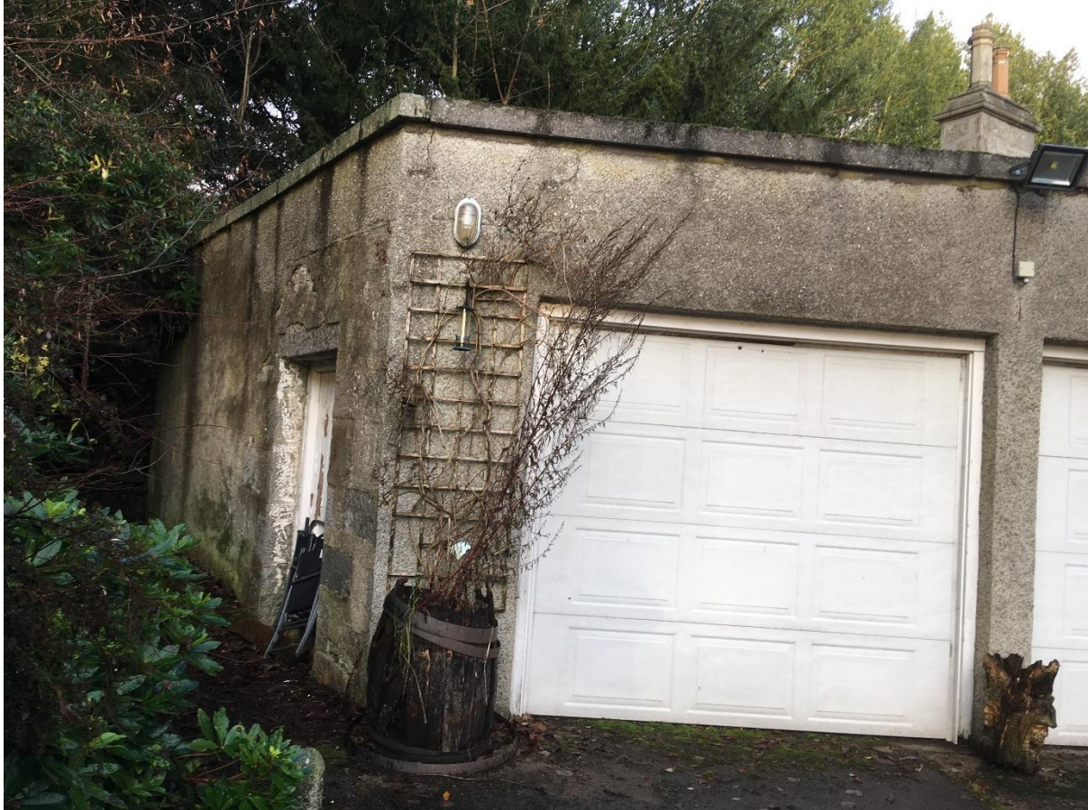
South and west elevations showing the garage door, modern access door, cement render and concrete cope
