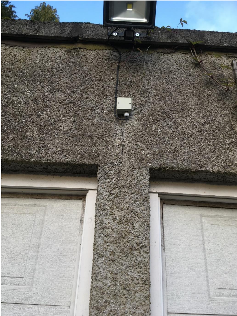
Cement harling, modern garage doors, modern concrete cope and light fitting to south elevation
