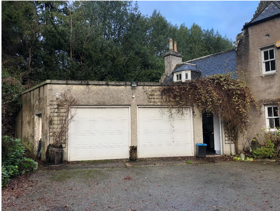
Front (south) Elevation with 20 th Century garage doors and pass door added
