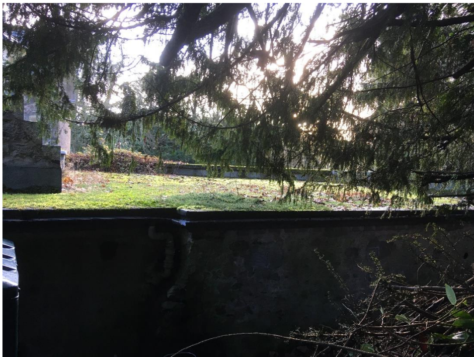
Rear (north) elevation is partially hidden, acting as a retaining wall to the adjacent ground
