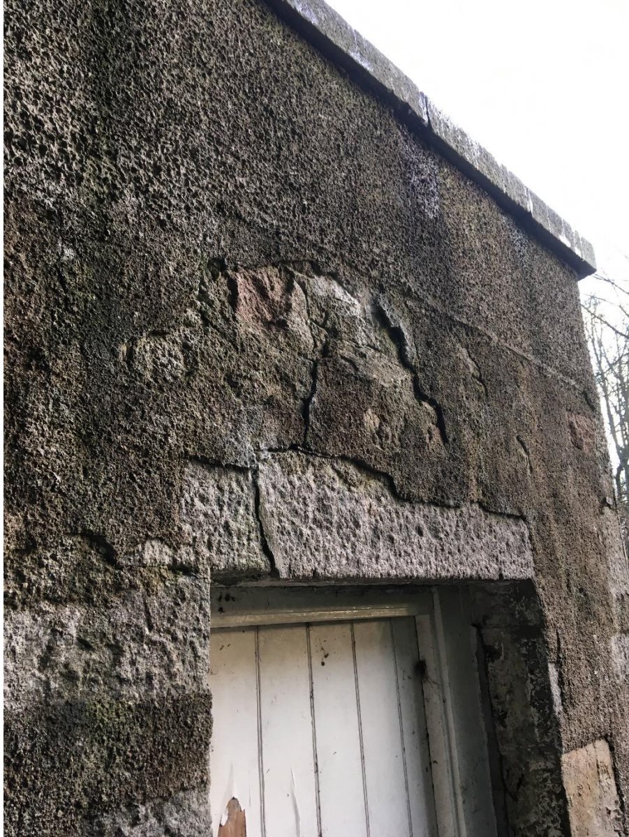
The cement harling is failing over parts of the extension (and main building)
