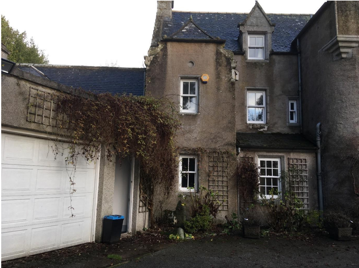
The south elevation of the extension connects back to the northernmost jerkin headed gable
