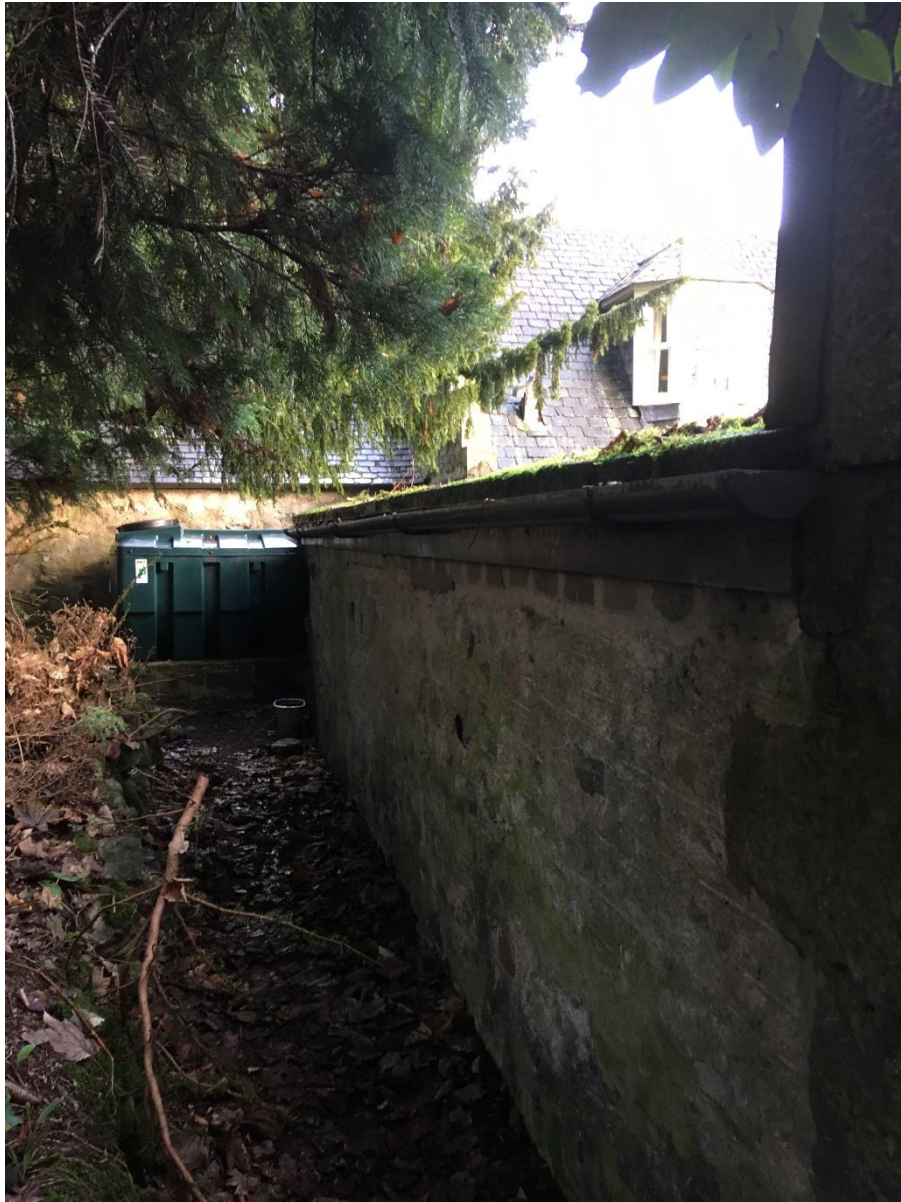
Rear (north) elevation is partially hidden, acting as a retaining wall to the adjacent ground
