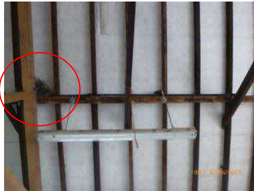
Figure 19. Birds' nests on the purlins and ridge board.
