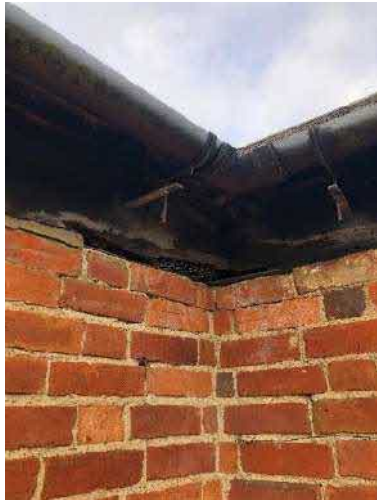
Figure 13. Gaps in wooden fascia.
