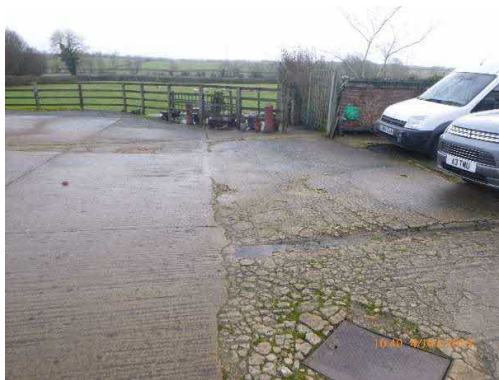
Figure 3. Cracks in hardstanding in places.
