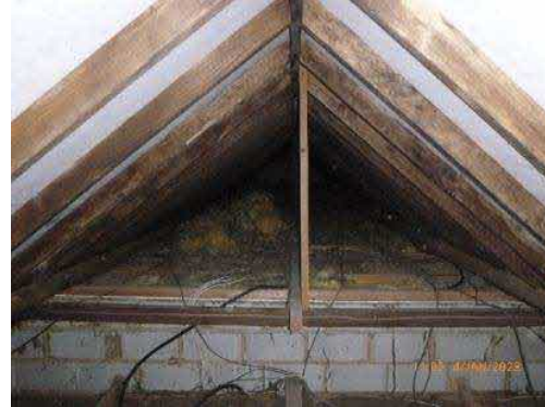
Figure 22. Concrete blocks and mineral wool insulation in roof voids.
