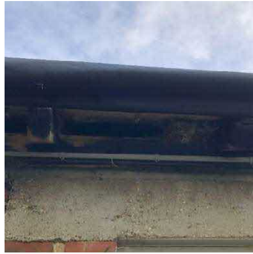
Figure 14. Missing fascia with birds' nest at eaves.
