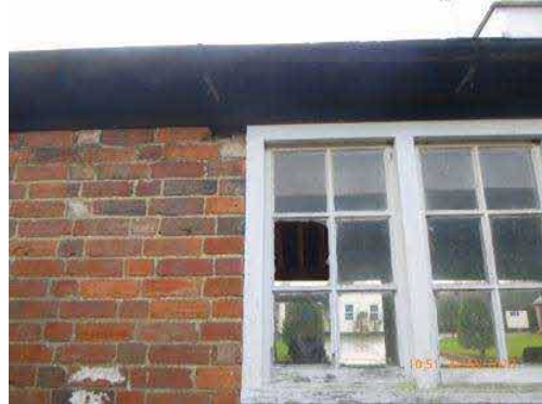
Figure 10. Wooden window frames and missing windowpane.
