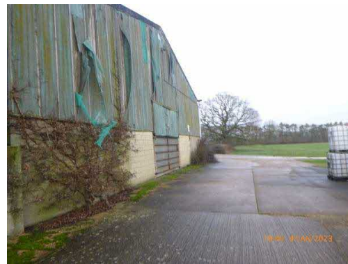
Figure 4. Moss and vegetation growing on hardstanding in places.
