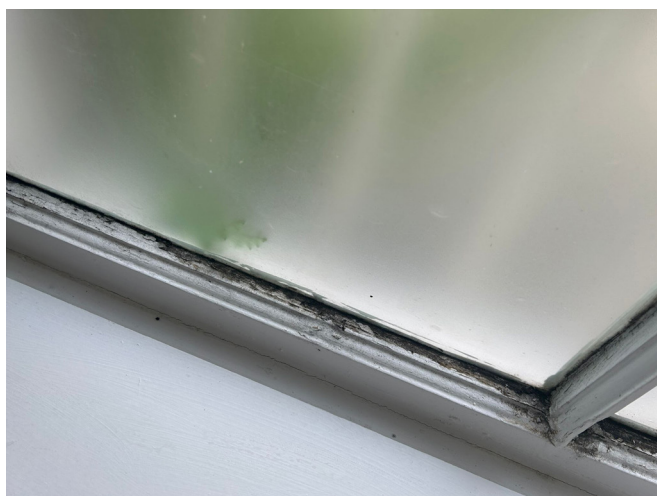
W1: Image from inside showing poor condition
