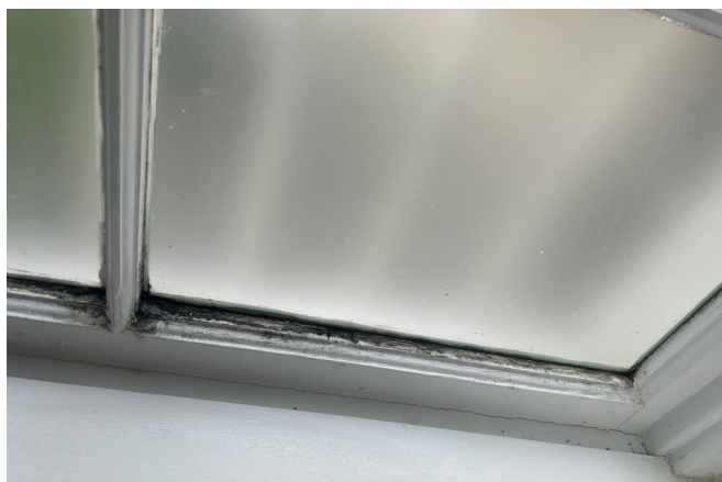
W2: Image from inside showing poor condition
