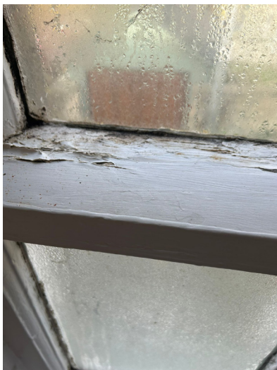
W4: Image showing poor condition
