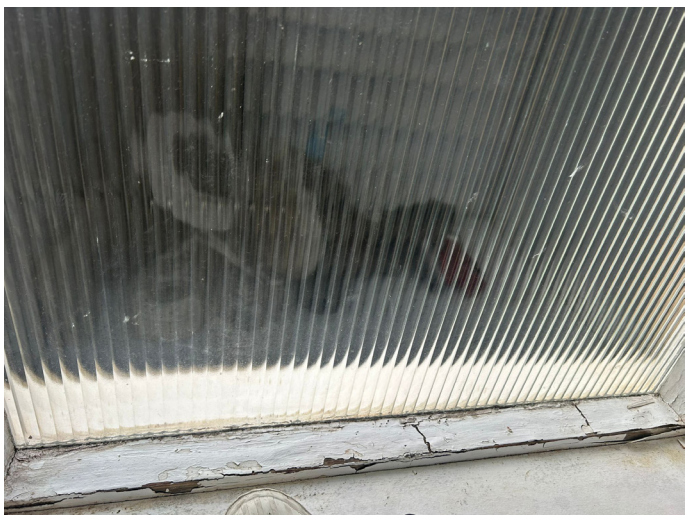
W6: Poor condition and non-original glazing
