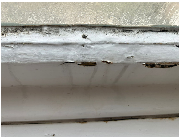
W5: Poor condition of timber, mould and condensation
