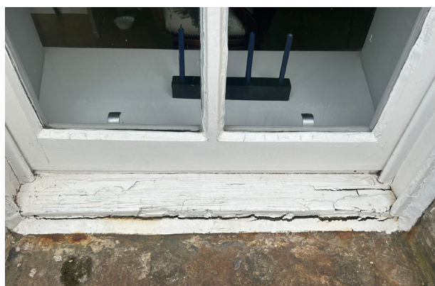
W10: Poor condition from exterior
