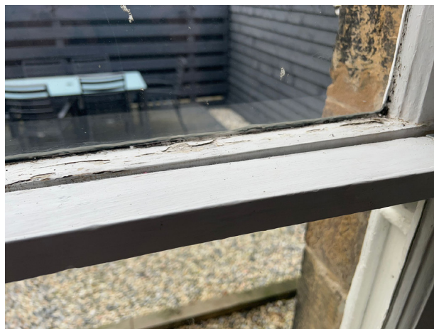
W7: Poor condition of sash and visible mould
