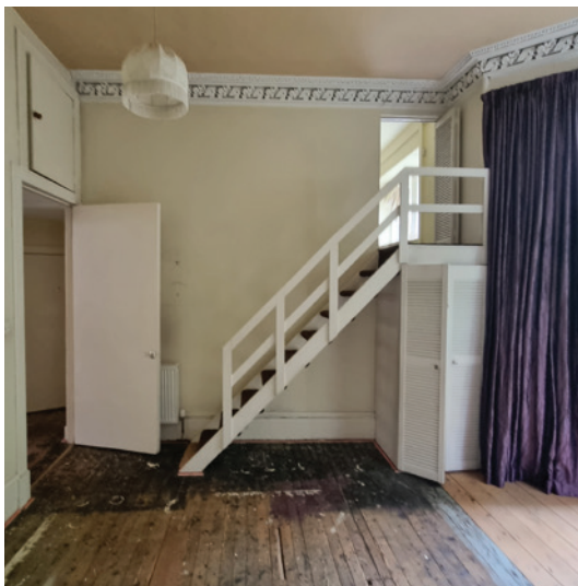
Stair to mezzanine with boiler cupboard
