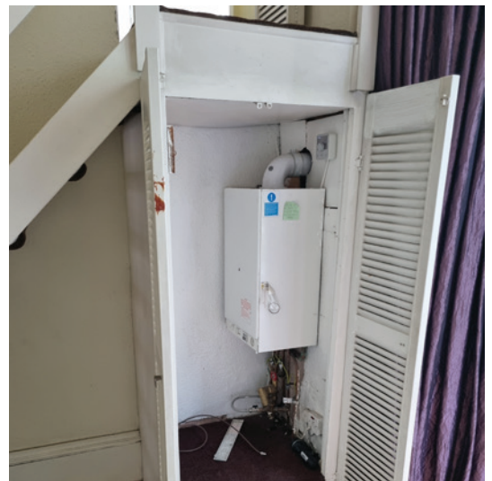
Boiler cupboard in bedroom
