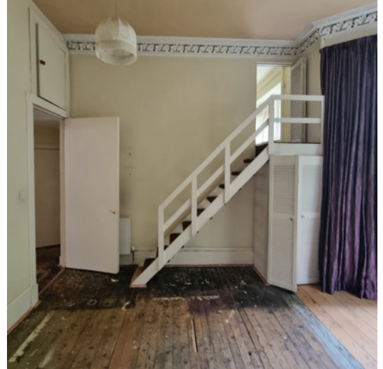
Stair to mezzanine with boiler cupboard
