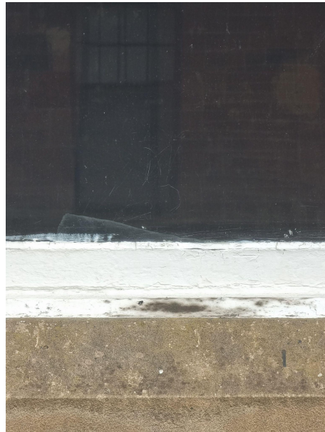
Signs of damp and rotting behind the mastic under the window.
