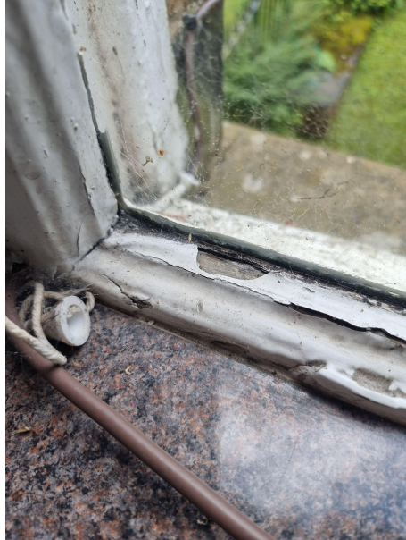
Bottom rail is showing signs of water damage and rot.
