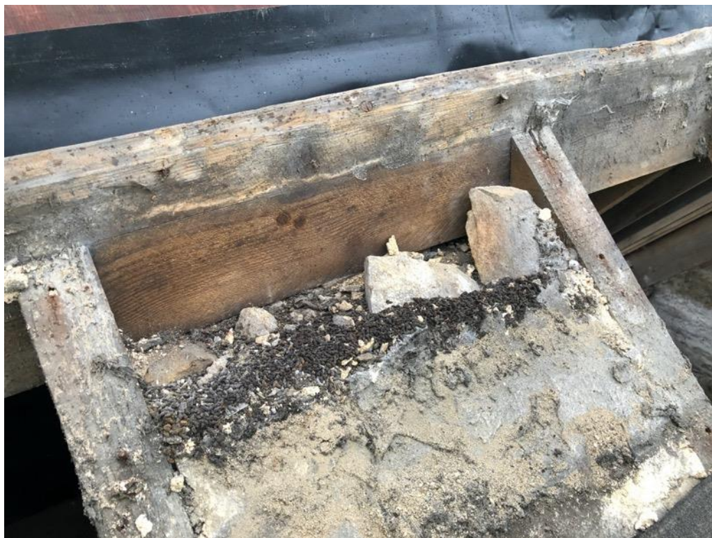
Plate 8: Example of bat droppings in eaves.
