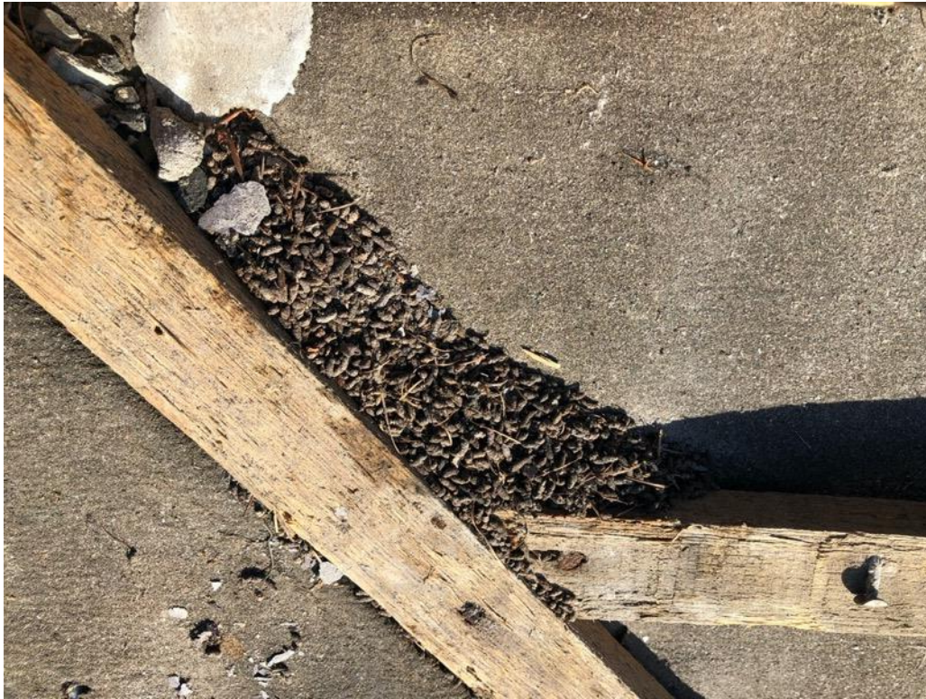
Plate 7: Example of bat droppings between slates (removed) and roof underlay, next to a roof valley.
