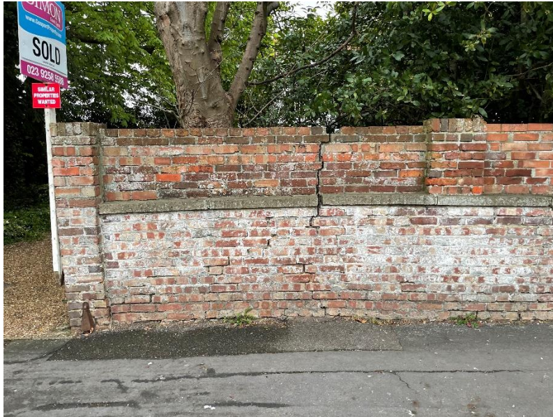
Existing Boundary Wall in Poor Condition
